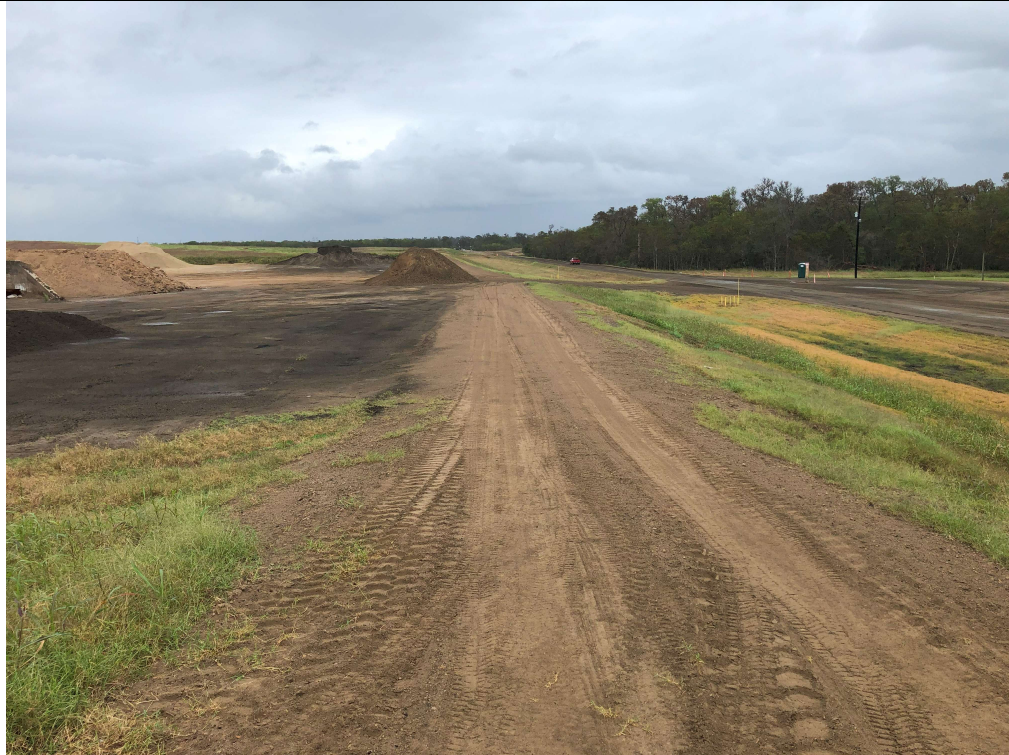
Photograph P-4: View looking north along the eastern edge of Cell 2A (the Pugmill Area). Stockpiled, salable CCR material is visible on the left side of this photograph.
