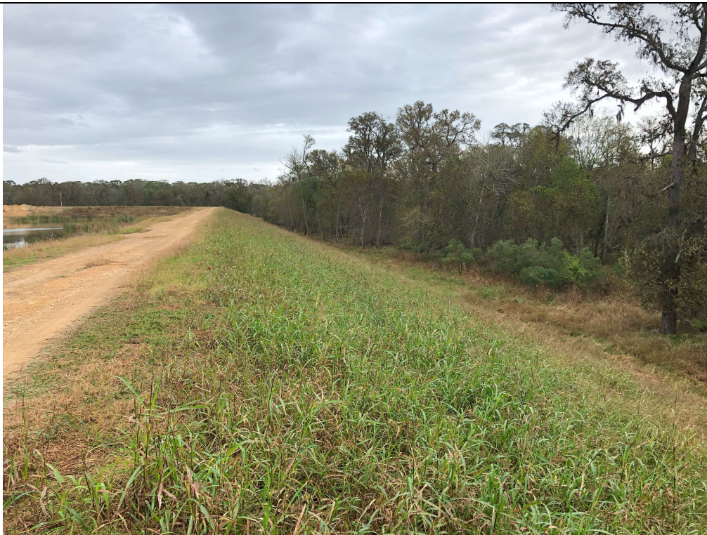
Photograph P-12: View looking southeast of the exterior slope of Cell 2B's southern berm. The exterior slope is well vegetated, stable, and not excessively steep. No erosional issues were observed.
