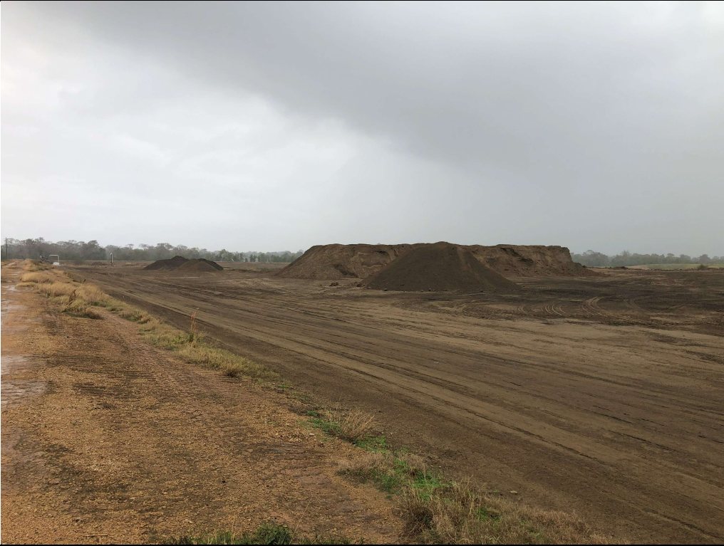
Photograph P-3: View looking northwest of the Cell 3 landfill and Cell 3 Coal Combustion Residual (CCR) waste piles. This material is being sold as road base.
