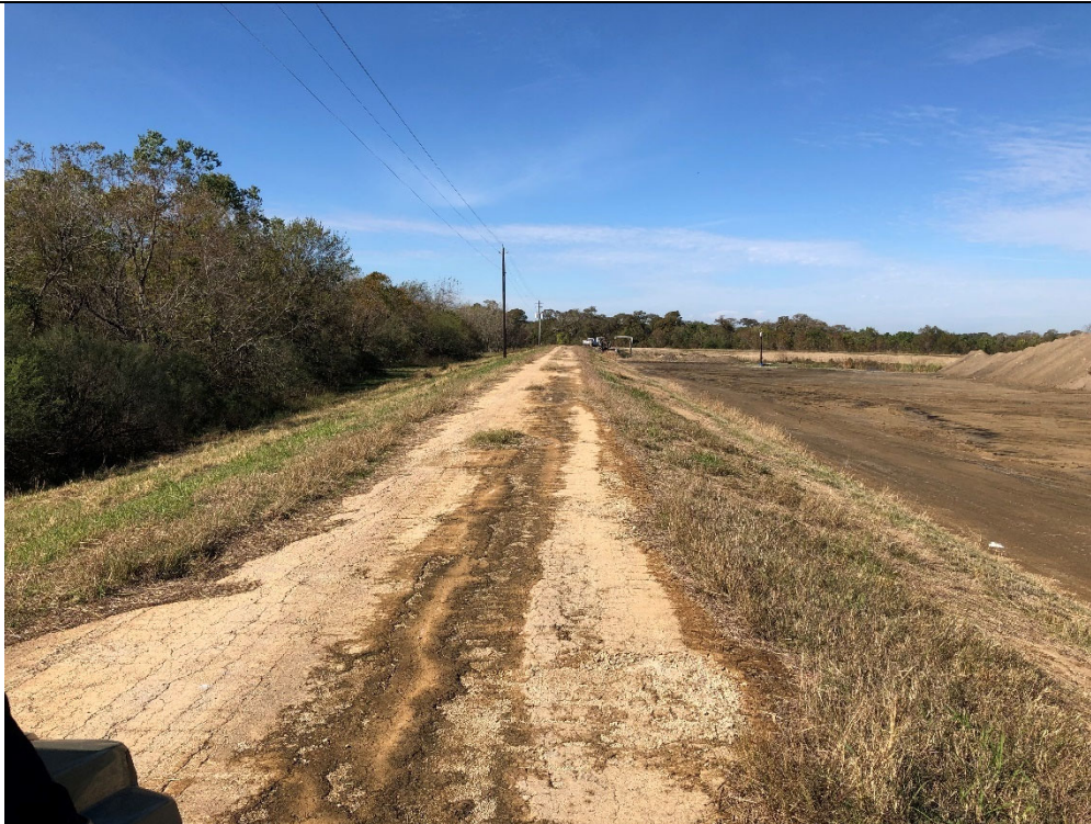
Photograph P-2: View looking west of Cell 3's south berm. The crest road was well maintained, exterior slopes well vegetated without erosion issues, and interior slope either improved with stabilized CCR material or vegetated.
