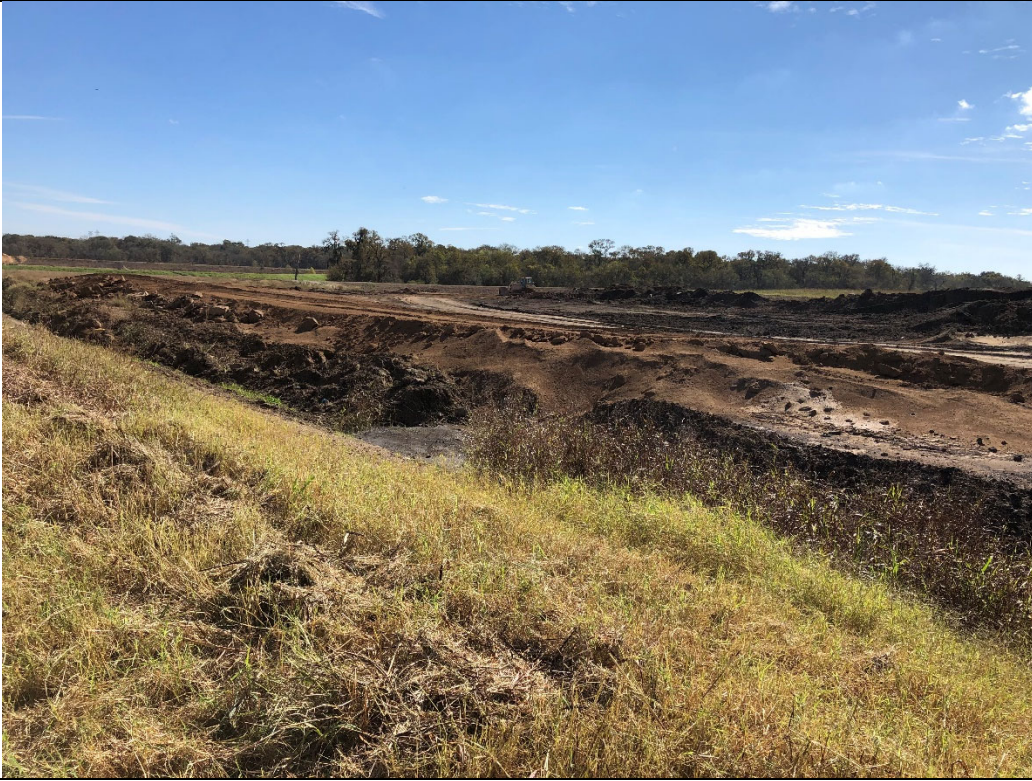
Photograph P-7: View looking northeast along the western berm of Cell 1C. Slopes were well stabilized. Although not visible, the crest road was stabilized with no significant rutting.
