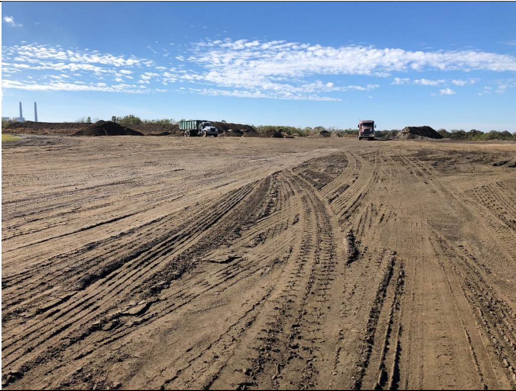
Photograph P-3: View looking west of interior of Cell 3 landfill and Cell 3 Coal Combustion Residual (CCR) waste piles. Trucks waiting to be loaded with salable bottom ash are visible in this photograph.
