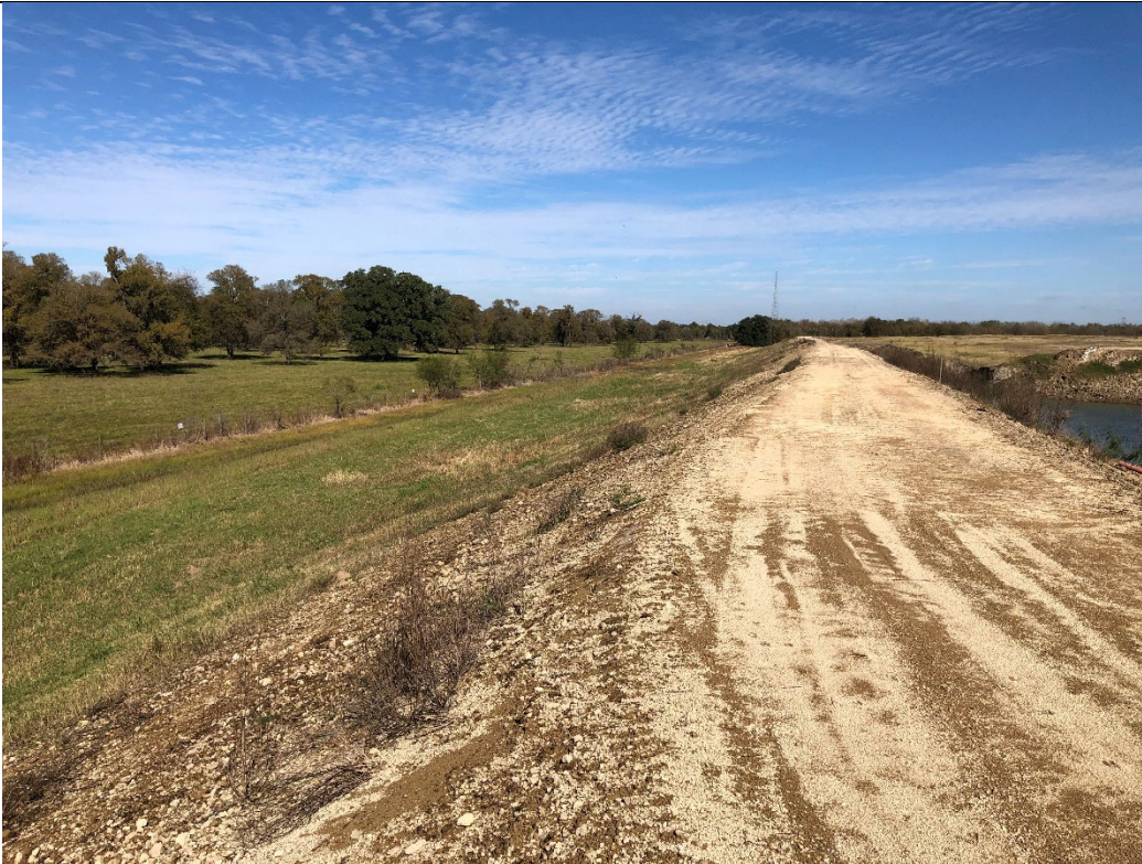
Photograph P-8: View looking north of the western berm of Cell 1C. The Cell 1C storm water pond is visible on the far right of this photograph.
