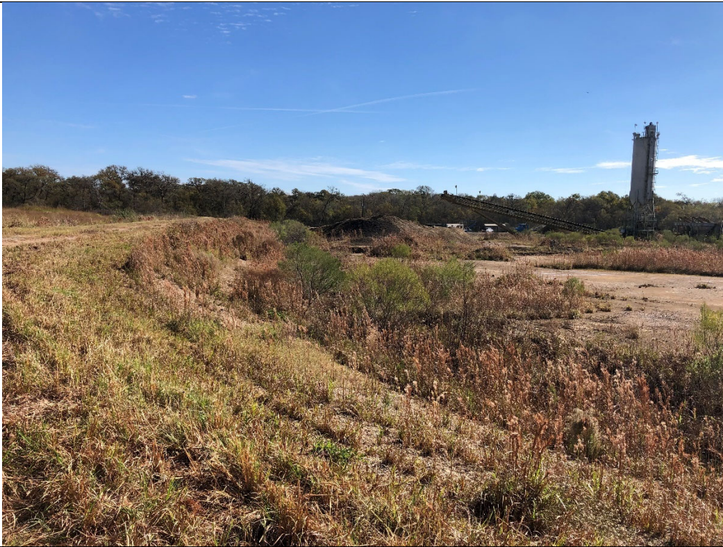
Photograph P-5: View looking east along the northern berm of Cell 2A, the Pugmill Area. Pugmill equipment and mixed CCR material are visible in this photograph.
