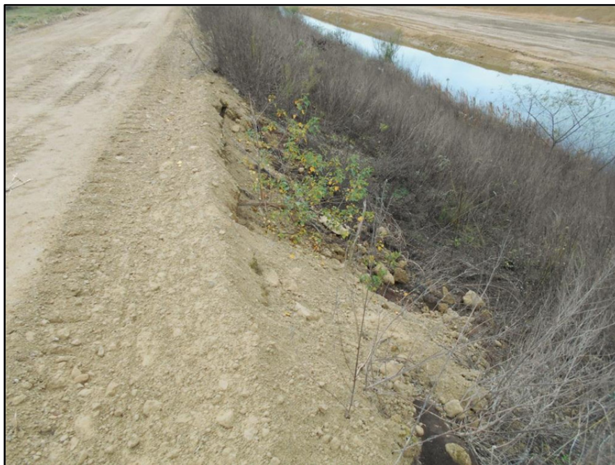
Photograph P-60 – Taken December 1, 2015 by David E. Nielson Landfill Cell 2B: Looking south along the inside slope of the eastern berm. Note the evidence of recent maintenance activities to protect the edge of the road.
