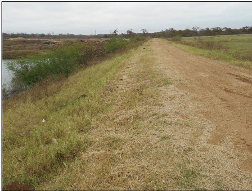
Photograph P-47 – Taken December 1, 2015 by David E. Nielson Landfill Cell 1C: Landfill Cell 1C: Looking east along the crest of the southern dike of the stormwater pond and then the western berm of the landfill.
