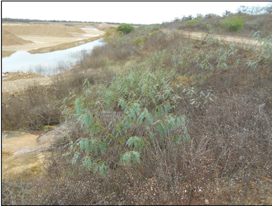
Photograph P-51 – Taken December 1, 2015 by David E. Nielson Landfill Cell 2B: Looking west along the inside slope of the northern berm. Note accumulation of stormwater.
