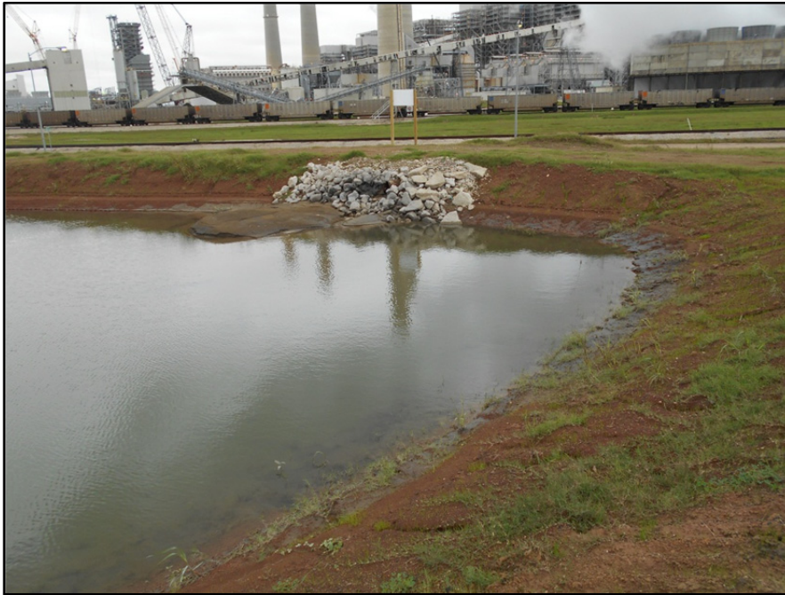
Photograph P-9 – Taken December 1, 2015 by David E. Nielson Air Preheater Pond: Looking north at northern inside slope of dike. Note the well armored area around the inlet pipe discharge into the pond that was not evident in Photograph P-6. The back of the required impoundment identification marker is shown beyond the riprap inlet. Also note the poor vegetative cover.
