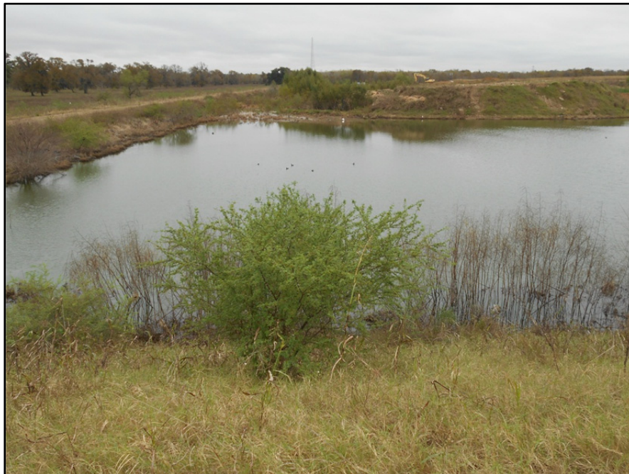
Photograph P-45 – Taken December 1, 2015 by David E. Nielson Landfill Cell 1C: Looking north along the inside slope of the western dike. Note small trees that should be removed.
