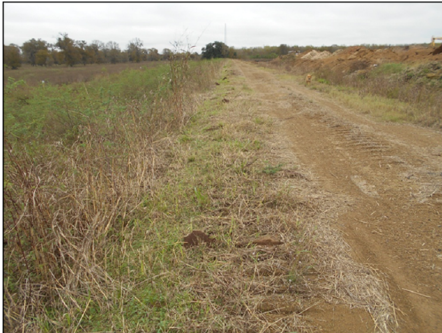
Photograph P-43 – Taken December 1, 2015 by David E. Nielson Landfill Cell 1C: Looking north along the outside crest of the western berm.
