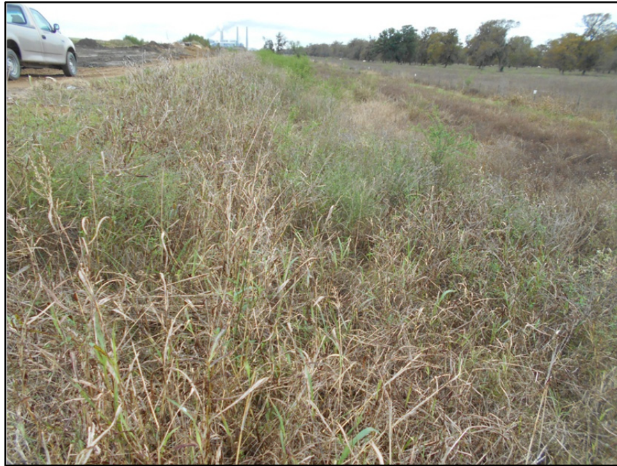
Photograph P-42 – Taken December 1, 2015 by David E. Nielson Landfill Cell 1C: Looking south along the outside slope of the western berm. Note vegetation control is warranted.
