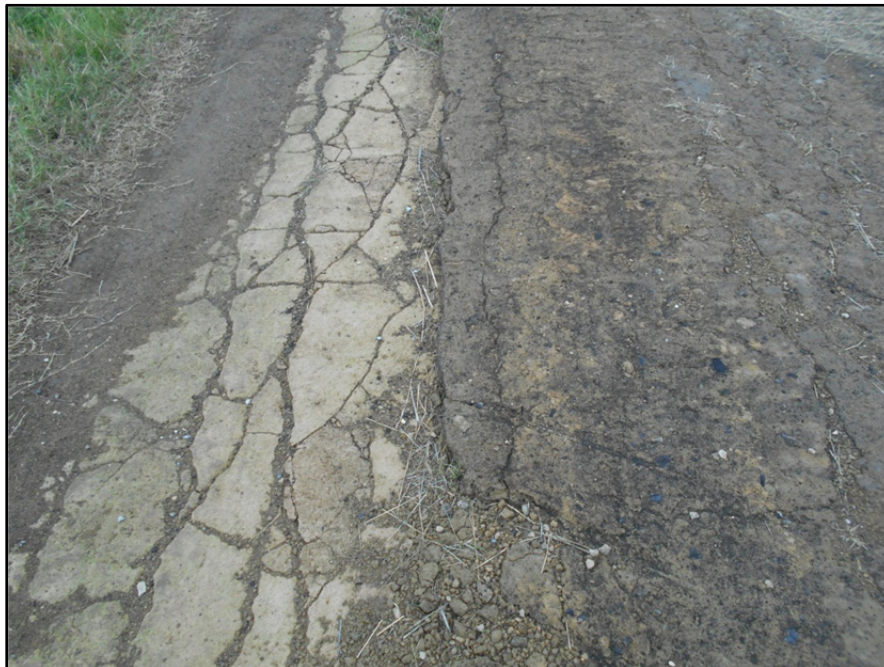
Photograph P-12 – Taken December 1, 2015 by David E. Nielson Landfill Cell 3: Looking west at the roadway along the crest of the landfill cell berm. Note the hard surfacing on this and other berm roads was a stabilized product that exhibited significant shrinkage cracks. These cracks are not indicative of berm instability.
