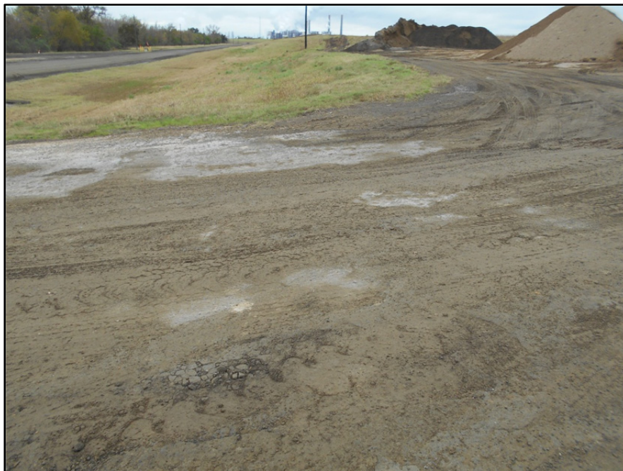
Photograph P-40 – Taken December 1, 2015 by David E. Nielson Landfill Cell 2A: Looking south at outside slope of the eastern berm.
