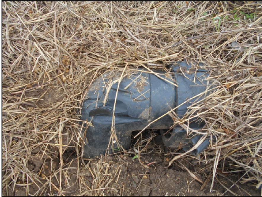
Photograph P-15 – Taken December 1, 2015 by David E. Nielson Landfill Cell 3: Looking at an exposed elbow of the discharge line from the stormwater pond. Note the damaged fitting appears to be from mowing equipment. This exposed fitting should be protected with bollards or buried after determination if it should be replaced.
