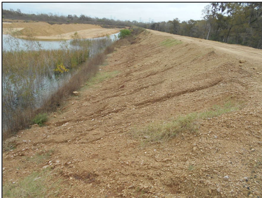
Photograph P-64 – Taken December 1, 2015 by David E. Nielson Landfill Cell 2B: Looking north along the inside slope of the landfill berm. Note ongoing erosion. Measures should be taken to mitigate erosion damage.
