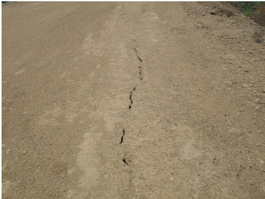
Photograph P-54 – Taken December 1, 2015 by David E. Nielson Landfill Cell 2B: Looking south along the road on the crest of the eastern berm. Note shrinkage crack in roadway surface material has been partially filled. See Photographs P-30 through P-33 and P-37 for other photographs of this type of crack. This is considered to be shrinkage of the stabilized road surface and not evidence of berm instability.
