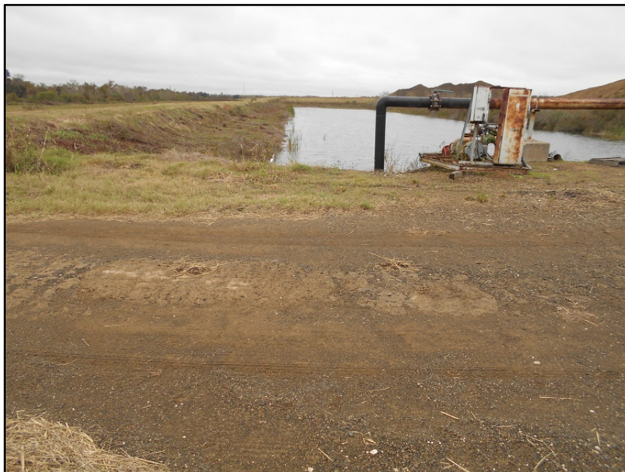
Photograph P-14 – Taken December 1, 2015 by David E. Nielson Landfill Cell 3: Looking north along the west dike of the stormwater pond in Cell 3 (also western extent of Cell 3) and the pump, which pumps water from the stormwater pond back to plant operations. Note some benching of the west dike of the pond. This appears to be the result of prior dredging activities to remove CCR material from the pond.
