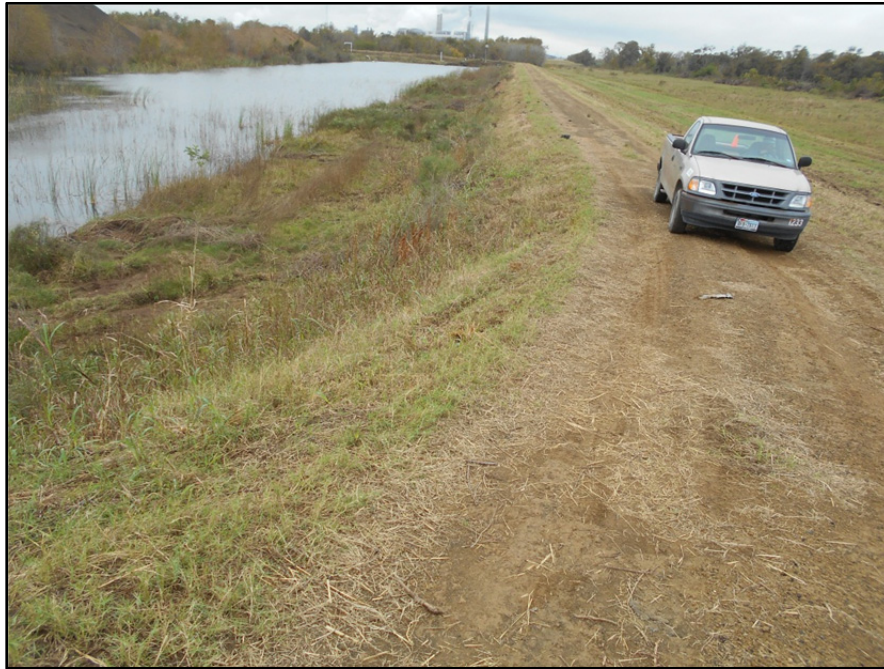
Photograph P-19 – Taken December 1, 2015 by David E. Nielson Landfill Cell 3: Looking south at inside slope of west dike of the stormwater pond and dike crest. Note it appears that significantly less CCR material is stored in the pond than is shown in Photograph P-10.
