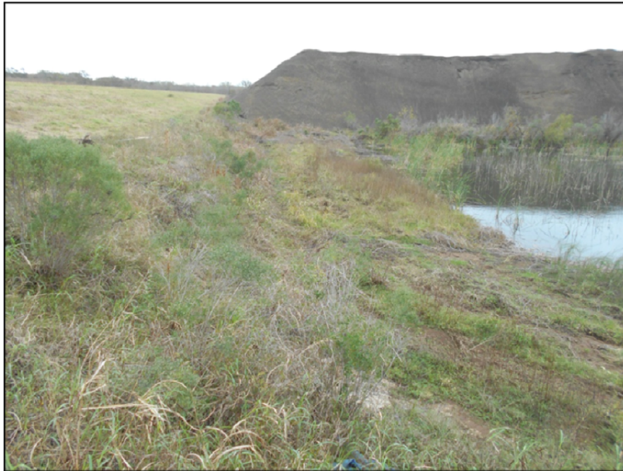
Photograph P-21 – Taken December 1, 2015 by David E. Nielson Landfill Cell 3: Looking east along inside slope of northern edge of pond, and at the interface of the ash storage area and the stormwater pond, which is incised relative to the closed landfill cell to the north.
