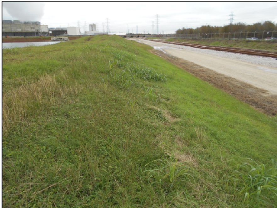
Photograph P-8 – Taken December 1, 2015 by David E. Nielson Air Preheater Pond: Looking northwest along the exterior slope of the eastern dike. Note good vegetation.
