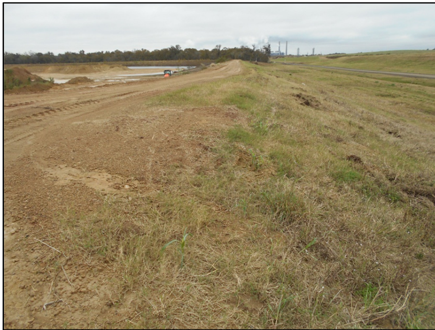
Photograph P-70 – Taken December 1, 2015 by David E. Nielson Landfill Cell 2B: Looking south along crest and outside slope of western berm/dike.
