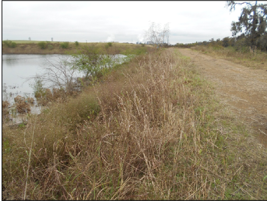
Photograph P-44 – Taken December 1, 2015 by David E. Nielson Landfill Cell 1C: Looking south along inside slope of western dike of stormwater pond. Note small trees that should be removed.
