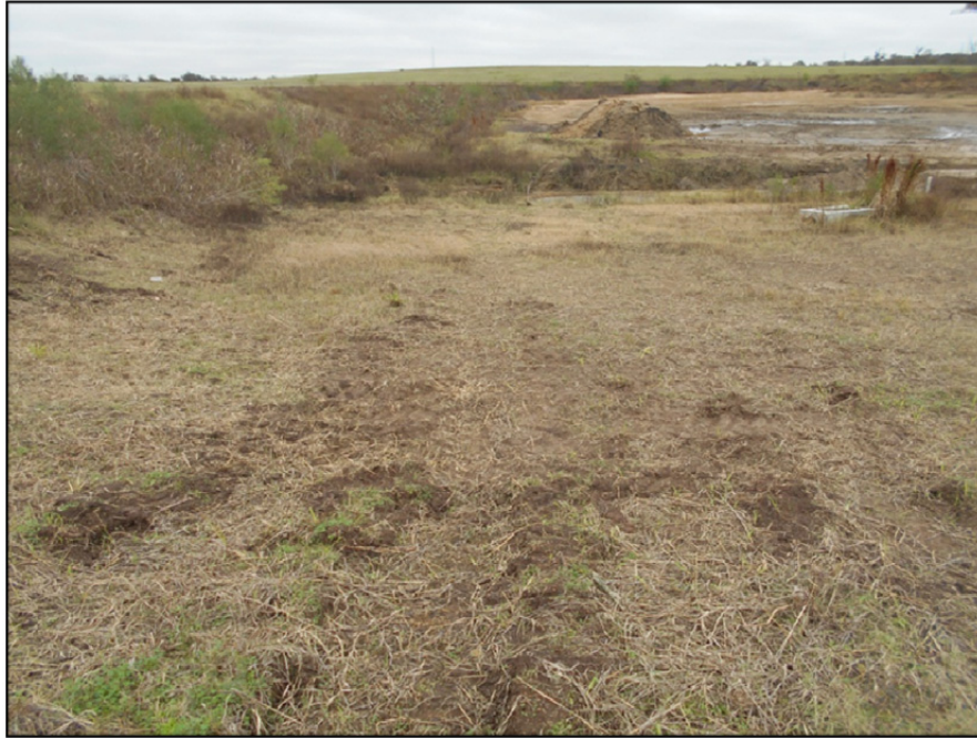
Photograph P-27 – Taken December 1, 2015 by David E. Nielson Landfill Cell 2A: Looking north along toe of inside slope of western berm.
