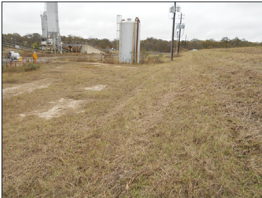
Photograph P-26 – Taken December 1, 2015 by David E. Nielson Landfill Cell 2A: Looking east along the inside slope of southern dike. Note large water tank in center of photograph is water storage for pugmill operations (inside cell in photograph background).
