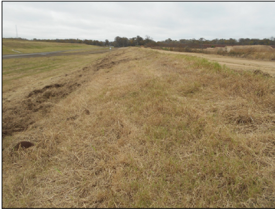
Photograph P-69 – Taken December 1, 2015 by David E. Nielson Landfill Cell 2B: Looking north along the exterior slope of the western dike/berm. Note uniformity of slope and generally good vegetation cover with feral hog damage near toe of slope.
