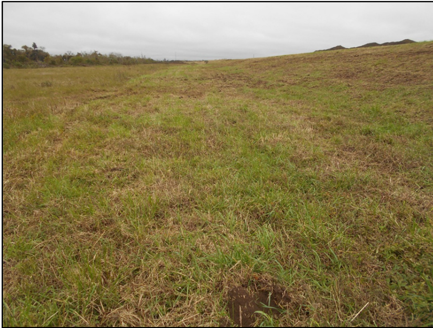
Photograph P-17 – Taken December 1, 2015 by David E. Nielson Landfill Cell 3: Looking north along outside slope of western dike of the stormwater pond. No instability or erosion was observed.
