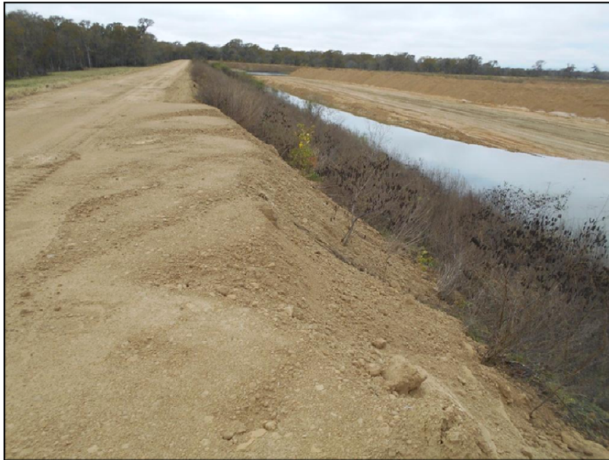
Photograph P-59 – Taken December 1, 2015 by David E. Nielson Landfill Cell 2B: Looking south along the inside slope of the eastern berm. Note the evidence of recent maintenance activities to protect the edge of the roadway and mitigate steep inside slopes.
