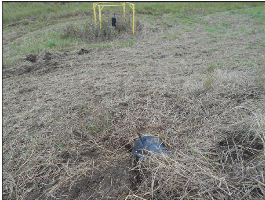
Photograph P-16 – Taken December 1, 2015 by David E. Nielson Landfill Cell 3: Looking west from the southwest corner of the landfill cell at the damaged fitting on the discharge pipe and valve control in the background.
