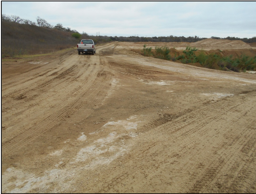
Photograph P-49 – Taken December 1, 2015 by David E. Nielson Landfill Cell 2B: Looking east along the crest of the northern berm. Note significant soil stockpile north of the berm crest.
