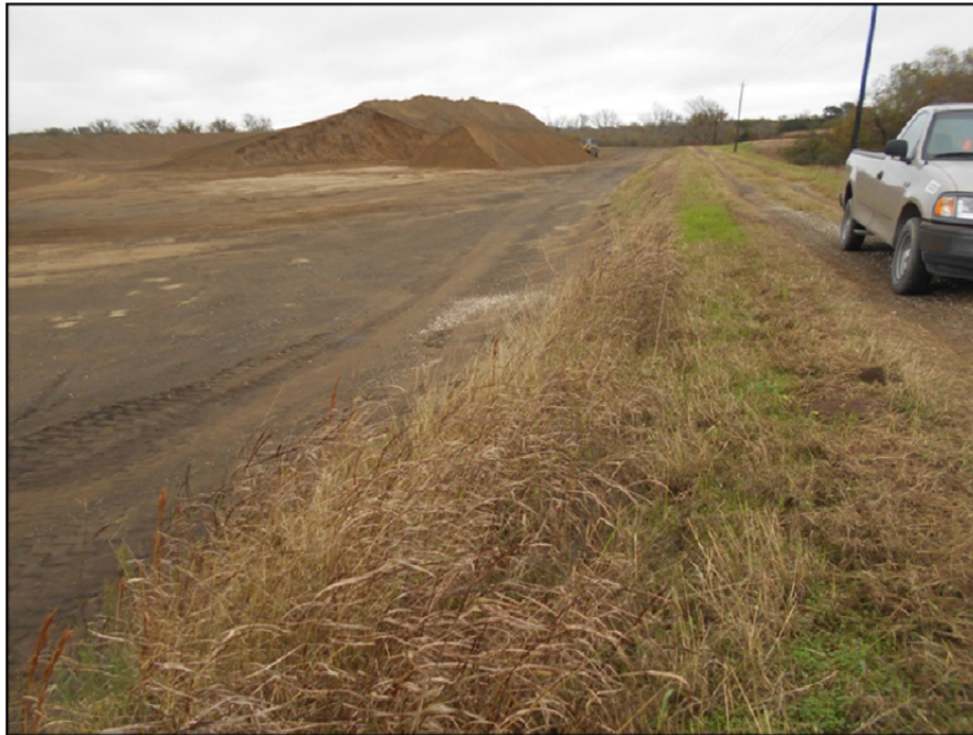
Photograph P-13 – Taken December 1, 2015 by David E. Nielson Landfill Cell 3: Looking east along the inside slope of the south berm.
