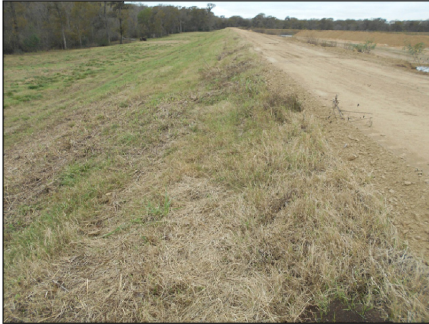
Photograph P-57 – Taken December 1, 2015 by David E. Nielson Landfill Cell 2B: Looking south along the crest of the outside slope of the eastern berm.
