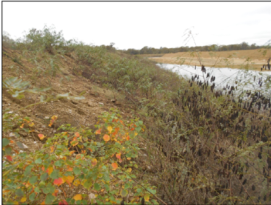
Photograph P-55 – Taken December 1, 2015 by David E. Nielson Landfill Cell 2B: Looking south along the inside slope of the eastern berm. Note vegetation irregularities and erosion.
