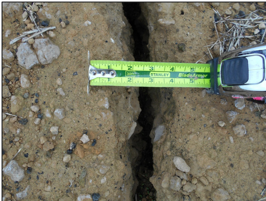
Photograph P-32 – Taken December 1, 2015 by David E. Nielson Landfill Cell 2A: Looking at wider than typical crack in stabilized roadway surfacing.
