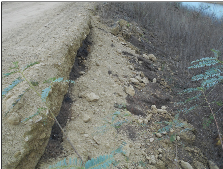
Photograph P-62 – Taken December 1, 2015 by David E. Nielson Landfill Cell 2B: Looking south along the inside slope of the eastern berm. Note sharp drop off at edge of road. This area should be protected from traffic near the edge of the road.
