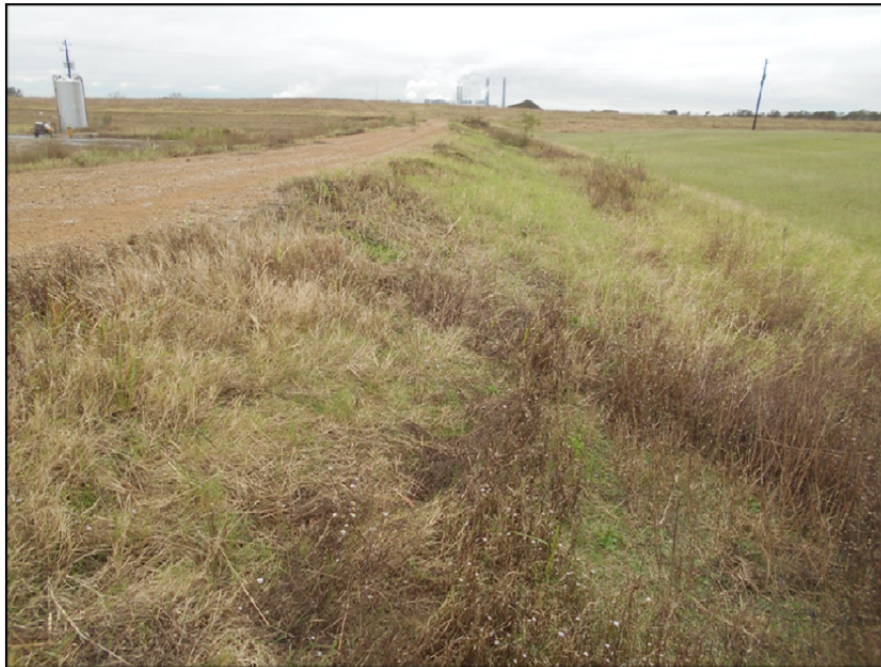
Photograph P-34 – Taken December 1, 2015 by David E. Nielson Landfill Cell 2A: Looking south along the outside face of the western berm.
