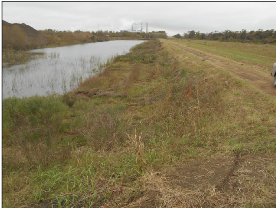
Photograph P-18 – Taken December 1, 2015 by David E. Nielson Landfill Cell 3: Looking south along inside slope of western dike of the stormwater pond. Benching appears to be a result of pond cleaning activities, not dike instability or wave erosion.
