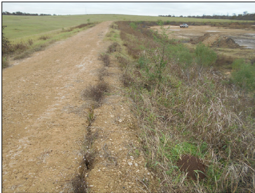
Photograph P-28 – Taken December 1, 2015 by David E. Nielson Landfill Cell 2A: Looking north along the crest of the western berm. Note closed sections of Cell 2A in background. Also note longitudinal crack in crest roadway surfacing.
