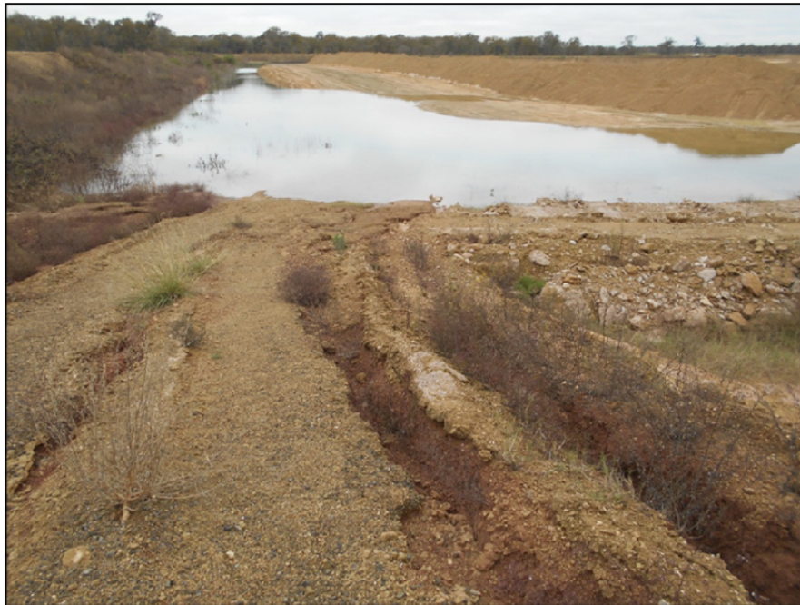
Photograph P-52 – Taken December 1, 2015 by David E. Nielson Landfill Cell 2B: Looking south along the inside slope and toe of slope of the eastern dike/berm.
