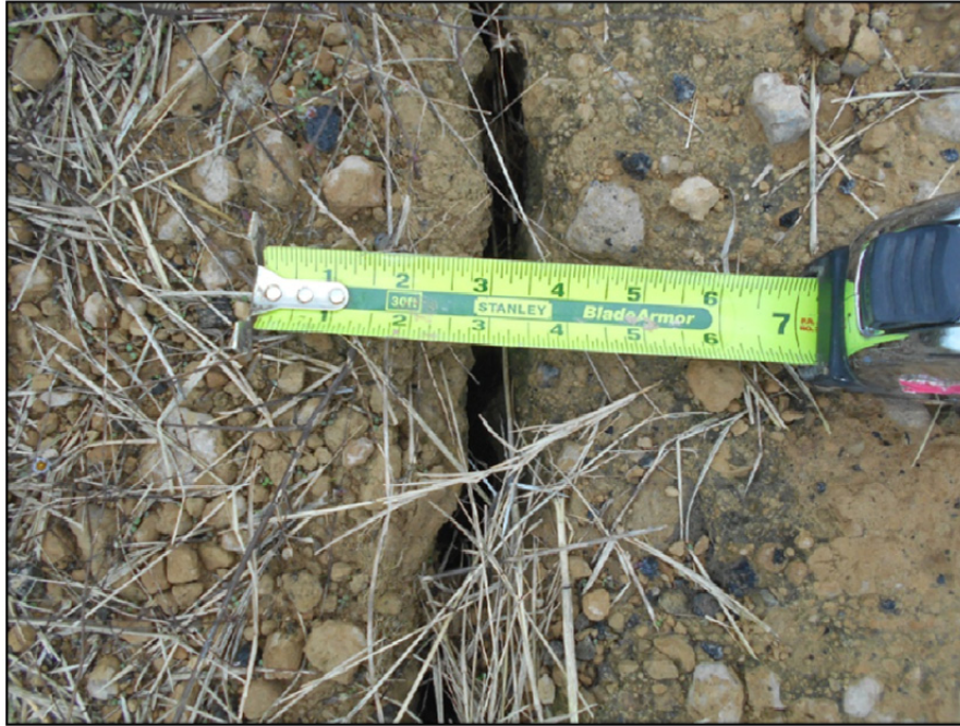
Photograph P-31 – Taken December 1, 2015 by David E. Nielson Landfill Cell 2A: Looking at typical crack in stabilized roadway surfacing.
