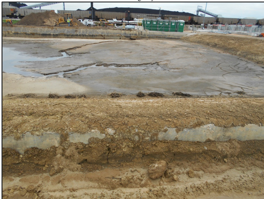
Photograph P-3 – Taken December 1, 2015 by David E. Nielson FGD Emergency Pond: Looking southwest at the western bank, which is incised. The dark horizontal line on the concrete wall in the background, as well as the level of the top of sediment in the right hand portion of the pond indicate the operating water level of the pond, which is well below the surrounding land surface (incised).
