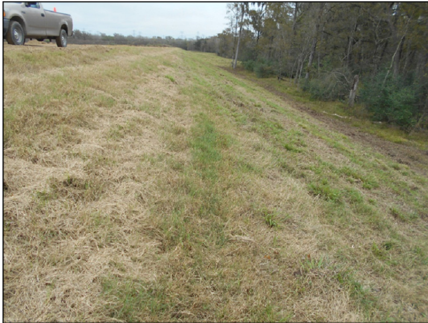
Photograph P-63 – Taken December 1, 2015 by David E. Nielson Landfill Cell 2B: Looking north along the outside slope of the eastern berm. Note generally good vegetation cover, uniform slopes and absence of erosion.
