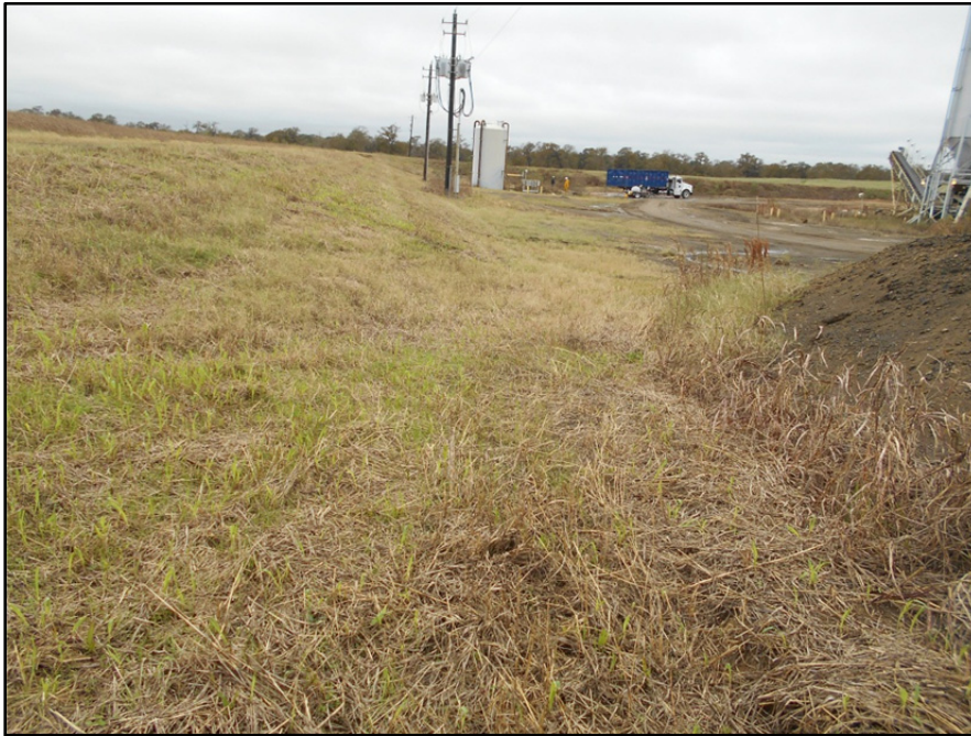
Photograph P-25 – Taken December 1, 2015 by David E. Nielson Landfill Cell 2A: Looking west along the inside slope of the southern berm. This berm abuts closed Cell 1B, which is higher in elevation. Note well established grass and uniformity of slope.
