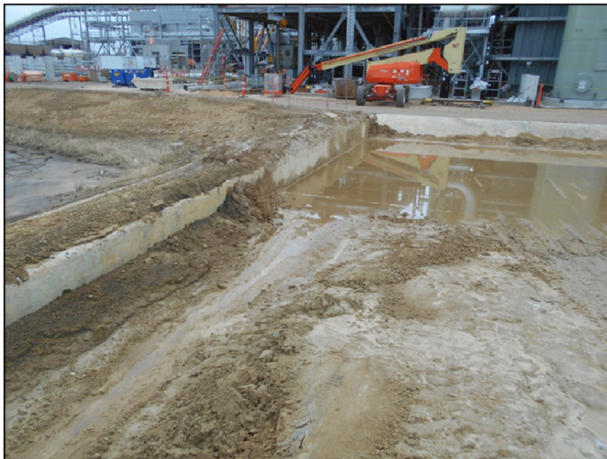
Photograph P-5 – Taken December 1, 2015 by David E. Nielson FGD Emergency Pond: Looking northwest at the junction of the northeast corner of FGD Emergency Pond and the adjacent depressed drainage slab, which is an incised area where excavated CCR materials are allowed to dry. This verifies that the Federal CCR Rule regarding inspections does not apply to the FGD Emergency Pond.
