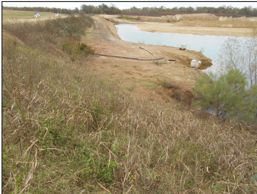
Photograph P-68 – Taken December 1, 2015 by David E. Nielson Landfill Cell 2B: Looking north along the inside slope of the west berm/dike at the area where a mobile pump is placed to remove stormwater collected in the cell. Note the slope is somewhat steep in the area of the ramp.
