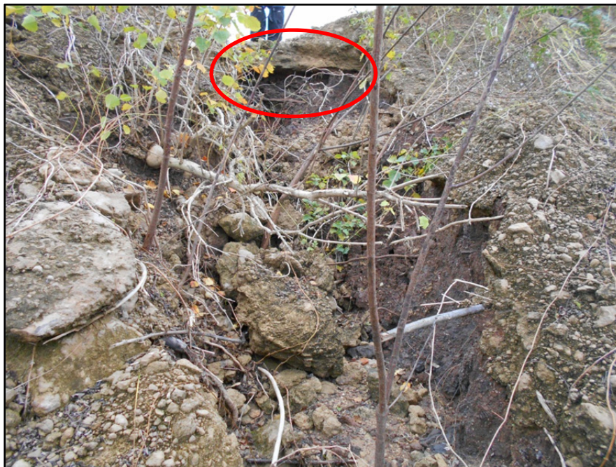
Photograph P-56 – Taken December 1, 2015 by David E. Nielson Landfill Cell 2B: Looking up at significant erosion of the inside slope of the eastern berm. Note the stabilized road surface has been undermined (circled in red). The disturbed soils should be removed, the erosional void should be backfilled and adequate erosion control measures should be implemented. In the interim, traffic should not be allowed near the edge of the roadway.
