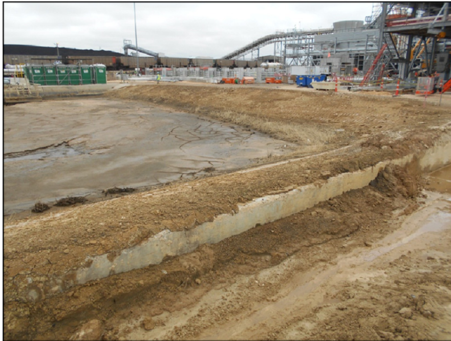
Photograph P-4 – Taken December 1, 2015 by David E. Nielson FGD Emergency Pond: Looking west at the northern end of FGD Emergency Pond, which is incised.
