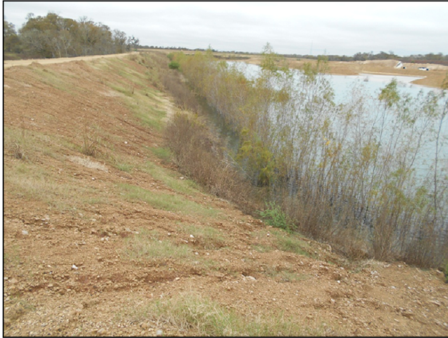
Photograph P-65 – Taken December 1, 2015 by David E. Nielson Landfill Cell 2B: Looking west along inside slope of southern berm/dike. Note sparse grass and small trees. Revegetation of slope is recommended.
