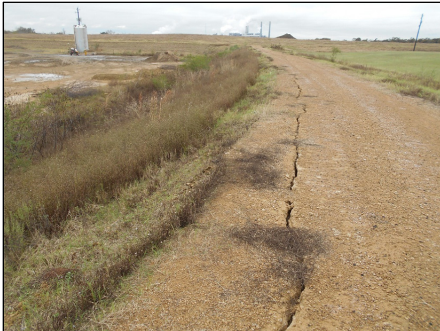
Photograph P-30 – Taken December 1, 2015 by David E. Nielson Landfill Cell 2A: Looking south along the inside slope and crest of western berm. Note significant crack in roadway surfacing. Cracks are also shown on Photographs P-31, P-32 and P-33. These cracks are not considered to be from shrinkage of the stabilized material not berm instability.
