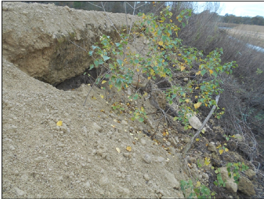
Photograph P-61 – Taken December 1, 2015 by David E. Nielson Landfill Cell 2B: Looking south along the inside slope of the eastern berm. Note undermining of the stabilized roadway and the steep nature of the inside slope.
