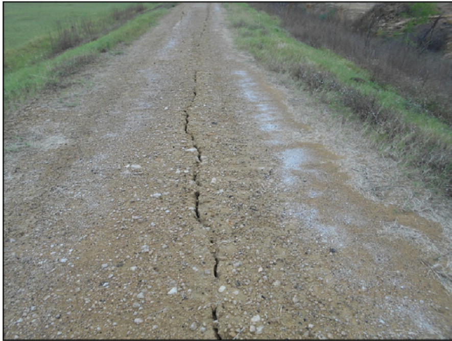
Photograph P-37 – Taken December 1, 2015 by David E. Nielson Landfill Cell 2A: Looking west along the northern dike crest. Note shrinkage crack in the road surfacing material.
