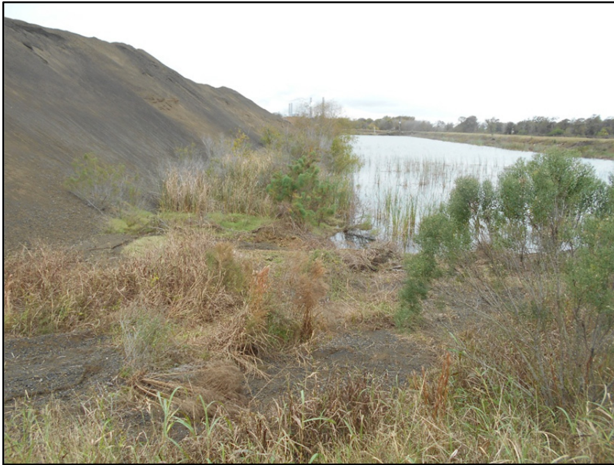
Photograph P-23 – Taken December 1, 2015 by David E. Nielson Landfill Cell 3: Looking south at inside slope of eastern boundary of stormwater pond and active landfill area.
