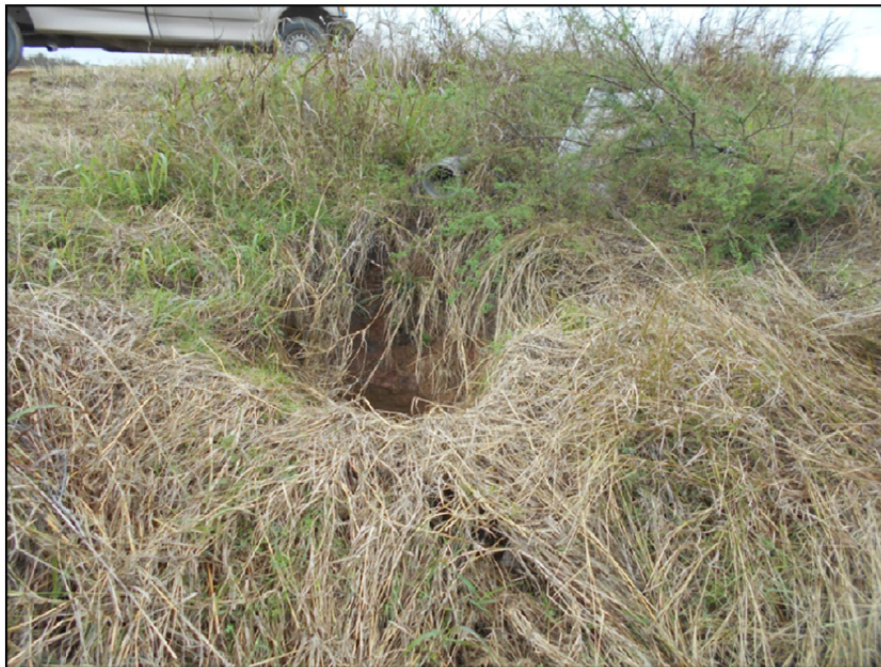
Photograph P-22 – Taken December 1, 2015 by David E. Nielson Landfill Cell 3: Looking north at discharge from stormwater pipe inlet into stormwater pond. Note the absence of a splash pad and the occurrence of erosion. The vegetation should be removed, the erosional void backfilled and a splash pad or other erosion control measure may be installed.
