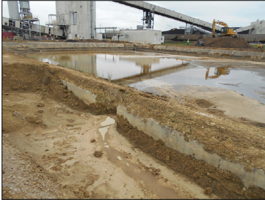
Photograph P-2 – Taken December 1, 2015 by David E. Nielson FGD Emergency Pond: Looking south at the southern and western banks, which are incised. This verifies that the Federal CCR Rule regarding inspections is not applicable to the FGD Emergency Pond.
