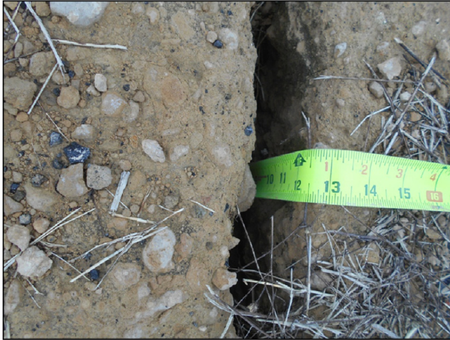
Photograph P-33 – Taken December 1, 2015 by David E. Nielson Landfill Cell 2A: Looking at wider than typical crack in stabilized roadway surfacing. The crack extended 1 foot below the roadway surface.
