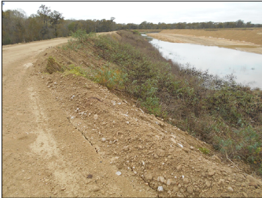
Photograph P-53 – Taken December 1, 2015 by David E. Nielson Landfill Cell 2B: Looking south along the inside slope of the eastern berm. Note crack formation along edge of the road and the steepness of some slope sections.
