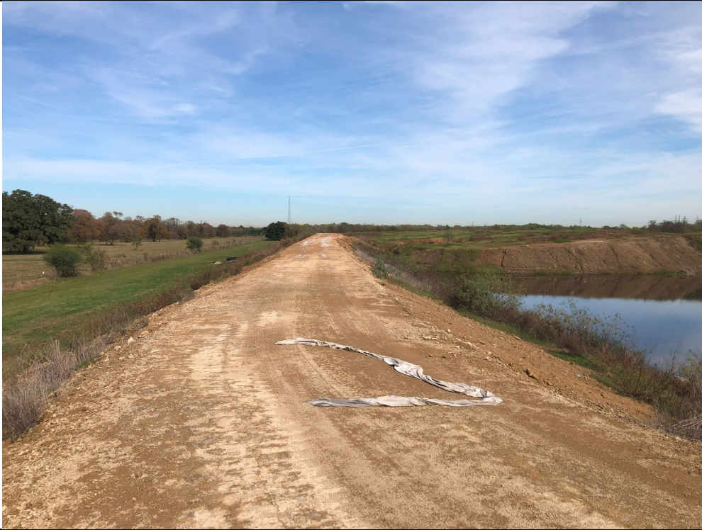
Photograph P-9: View looking north along the western berm of Cell 1C. Picture was taken from berm at southwest corner of Cell 1C. No significant rutting was observed.
