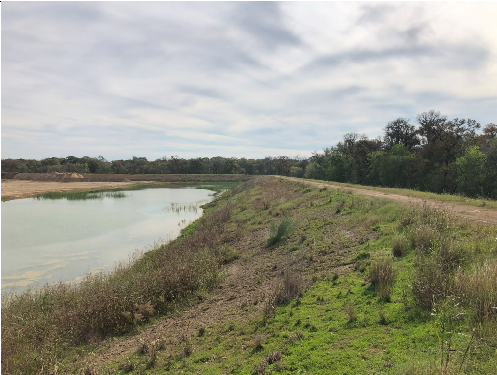
Photograph P-12: View looking southeast of Cell 2B's southern berm from southwest corner of landfill. The Cell 2B stormwater pond is visible to the left.
