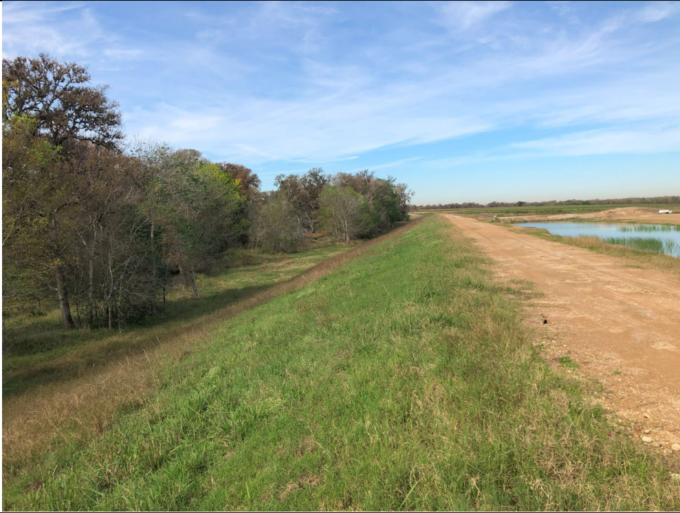
Photograph P-13: View looking northwest of the exterior slope of Cell 2B's southern berm. The exterior slope is well vegetated.
