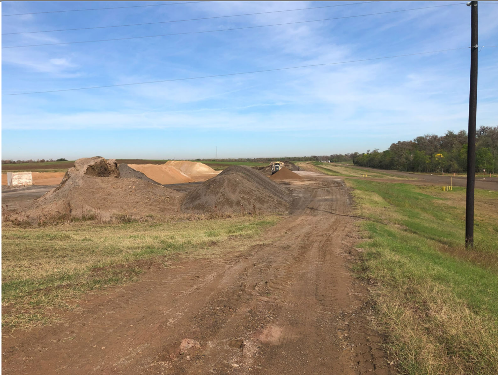
Photograph P-4: View looking north along the eastern edge of Cell 2A (the Pugmill Area). Stockpiled, salable CCR material is visible in this photograph.
