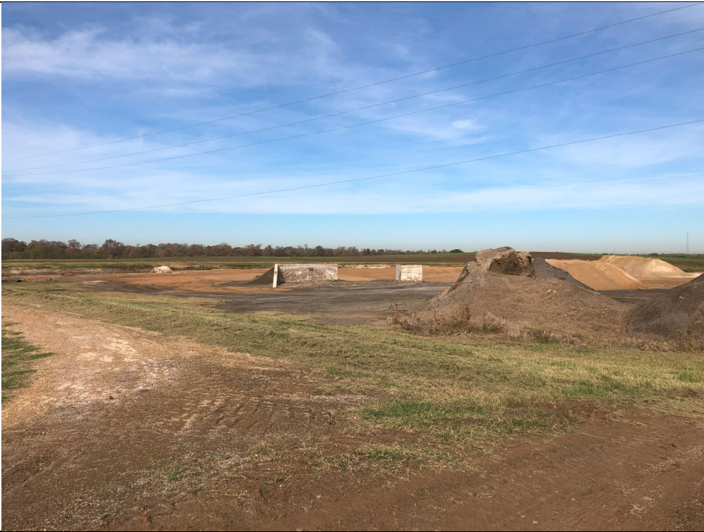
Photograph P-5: View looking northwest from the eastern edge of Cell 2A. Stockpiles of salable CCR material are visible in this photograph.
