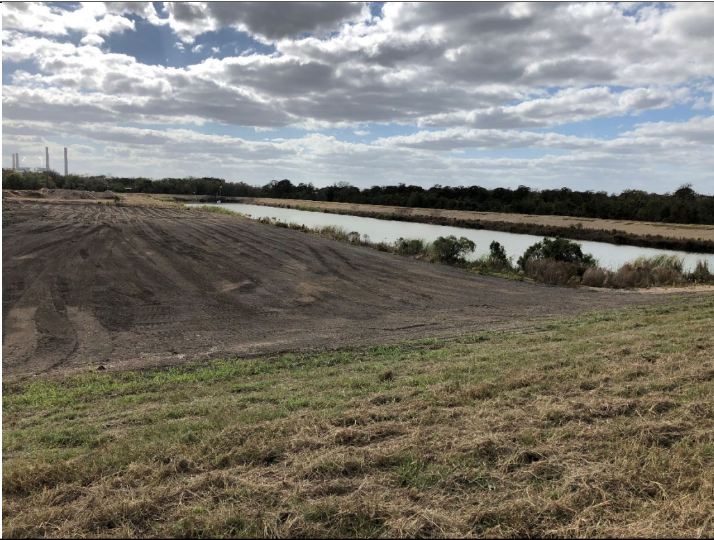
Photograph P-1: View looking south-southwest of Cell 3 from top of north berm. Bottom ash material is visible to the left; the Cell 3 contact water pond to the right. The interior slopes and crest roads of the berms have been stabilized with a cemented mixture of bottom ash and fly ash. The remainder of the berms are well vegetated.
