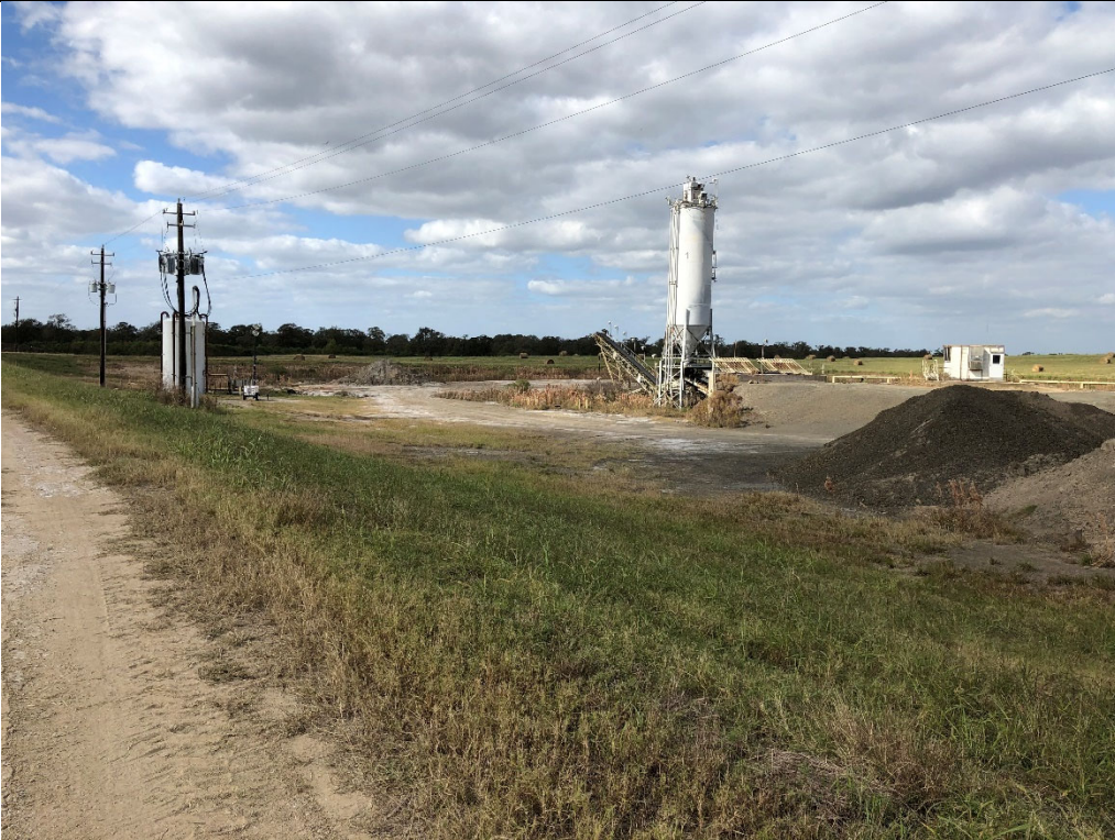
Photograph P-4: View looking west along the south berm of Cell 2A (the Pugmill Area).
