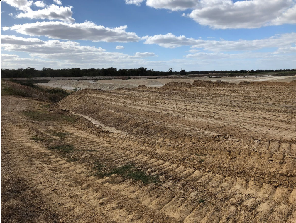
Photograph P-11: View looking southwest of Flue Gas Desulfurization (FGD) waste interred on north side of Cell 2B. This photograph was taken from the northeast corner of the landfill. The fly ash storage area is visible in the center background (beyond the FGD waste).
