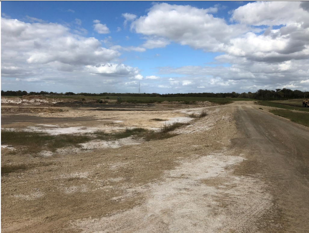
Photograph P-7: View looking north along the eastern berm of Cell 1C. Slopes were either stabilized (interior) or well vegetated (exterior). Crest road was stabilized with no significant rutting.
