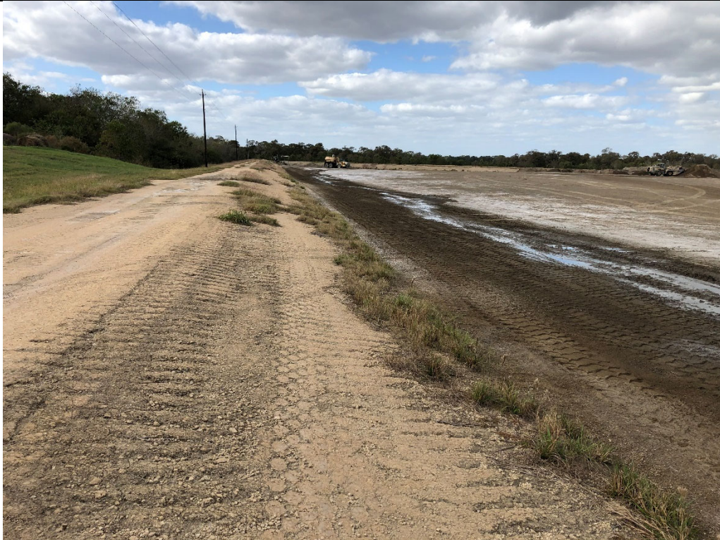
Photograph P-2: View looking west of Cell 3's south berm. The crest road was well maintained, exterior slopes well vegetated without erosion issues, and interior slope improved with stabilized CCR material.
