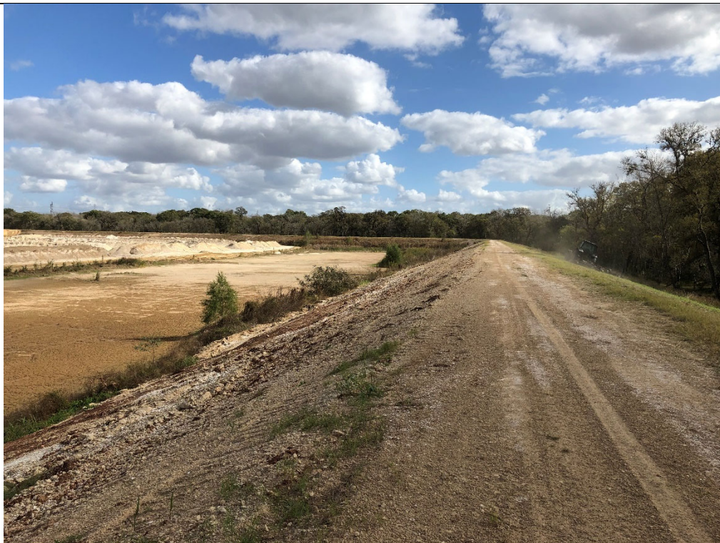
Photograph P-12: View looking east of Cell 2B's southern berm. The section of the interior slope of the southern berm that was recently repaired is visible on in this photograph (left foreground). The contact water pond is visible in the left background. The crest road and vegetated exterior slope are visible in the center and right sides of the photograph.
