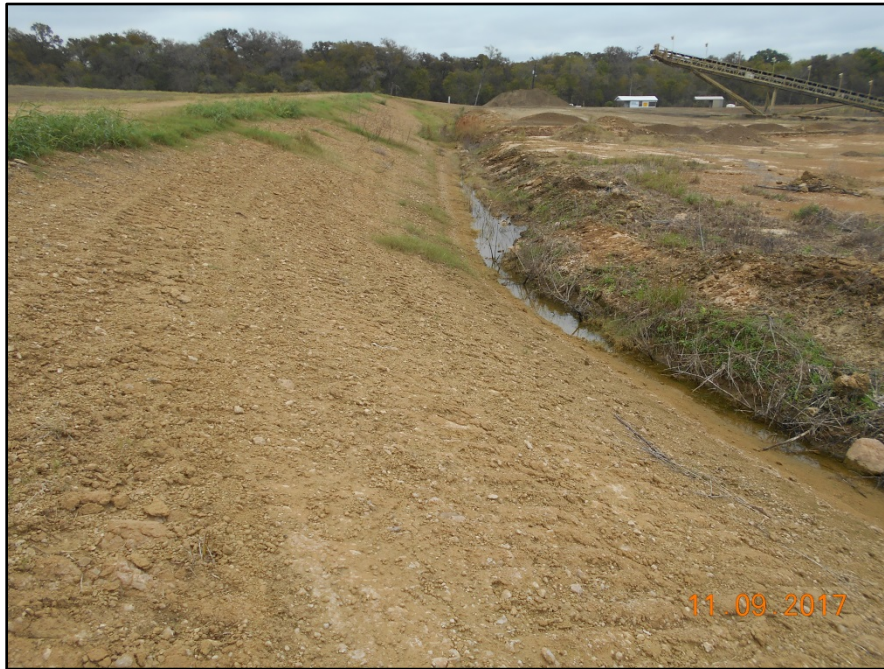
Photograph P-19 – Taken November 9, 2017 by David E. Nielson Landfill Cell 2A: Looking east along the inside slope of northern berm.
