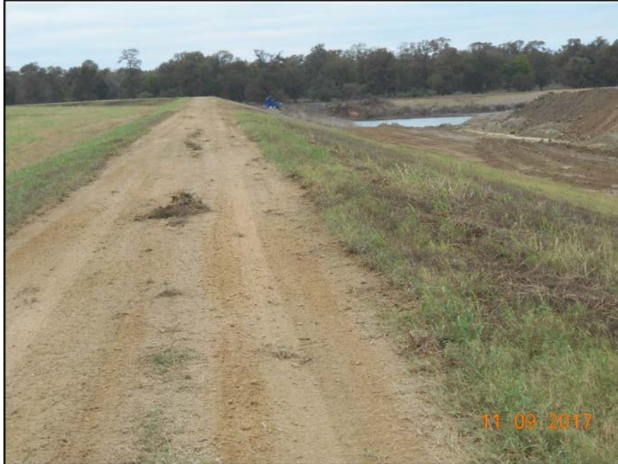
Photograph P-24 – Taken November 9, 2017 by David E. Nielson Landfill Cell 1C: Looking west along the crest of the southern berm of the cell with a view of the incised storm water pond.
