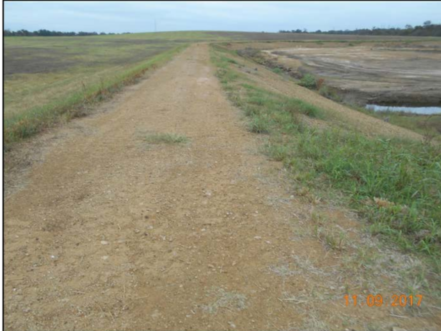
Photograph P-15 – Taken November 9, 2017 by David E. Nielson Landfill Cell 2A: Looking north along the crest of the western berm.
