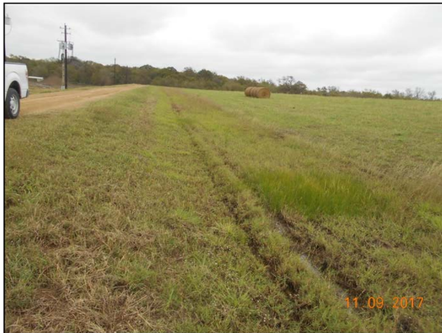
Photograph P-14 – Taken November 9, 2017 by David E. Nielson Landfill Cell 2A: Looking east along the crest and outside slope of southern dike.
