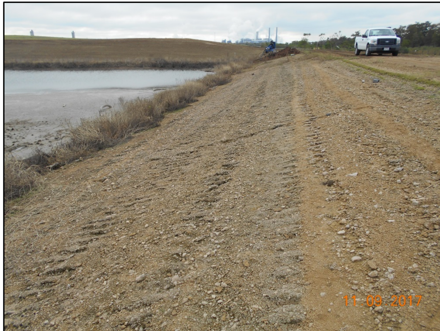
Photograph P-27 – Taken November 9, 2017 by David E. Nielson Landfill Cell 1C: Looking south along the inside slope of the western landfill cell berm.
