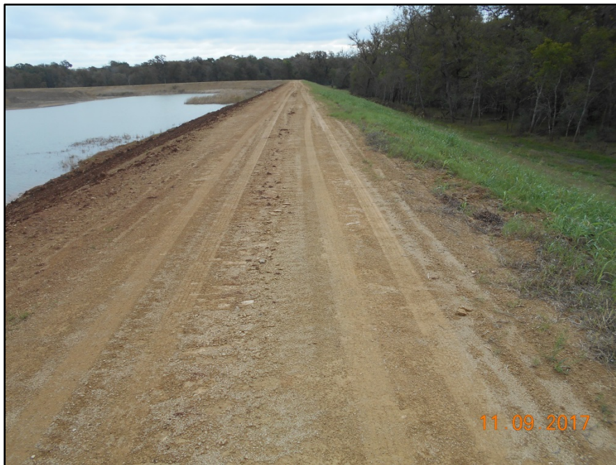
Photograph P-48 – Taken November 9, 2017 by David E. Nielson. Landfill Cell 2B: Looking east along the crest of southern berm.
