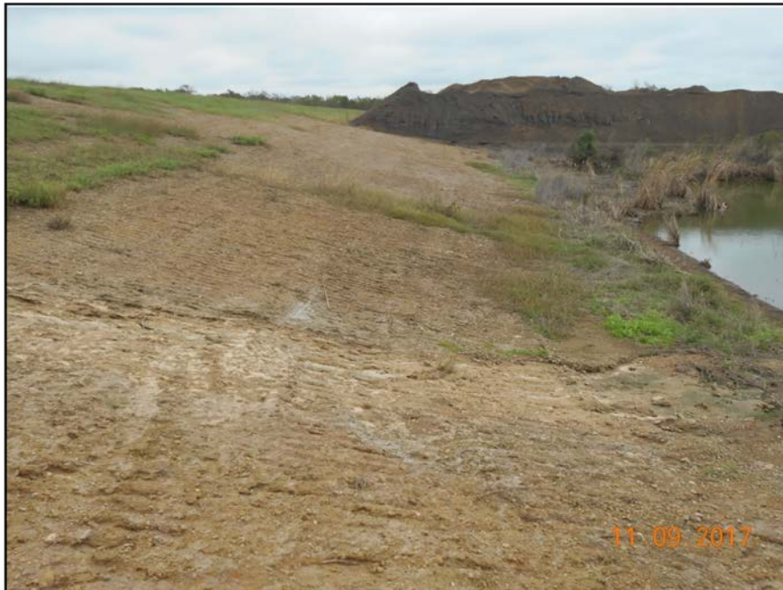
Photograph P-9 – Taken November 9, 2017 by David E. Nielson Landfill Cell 3: Looking east along inside slope of northern edge of pond, and at the interface of the ash storage area and the storm water pond, which is incised.
