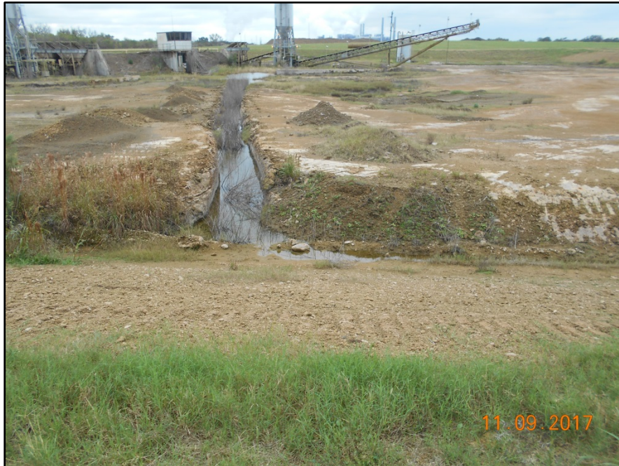
Photograph P-21 – Taken November 9, 2017 by David E. Nielson Landfill Cell 2A: Looking south into the active portion of Cell 2A along a vertical wall ditch cut in the stabilized material that has cured in place. These vertical walls demonstrate the long-term properties of these stabilized CCR materials.
