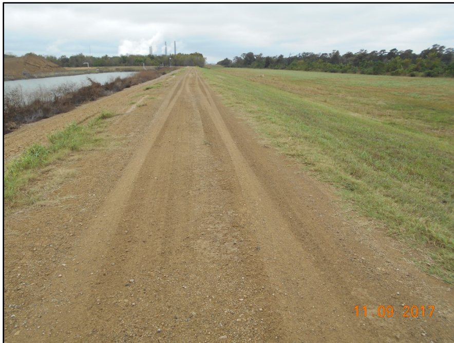
Photograph P-7 – Taken November 9, 2017 by David E. Nielson Landfill Cell 3: Looking south along crest of the western berm of the landfill cell in vicinity of incised storm water pond.
