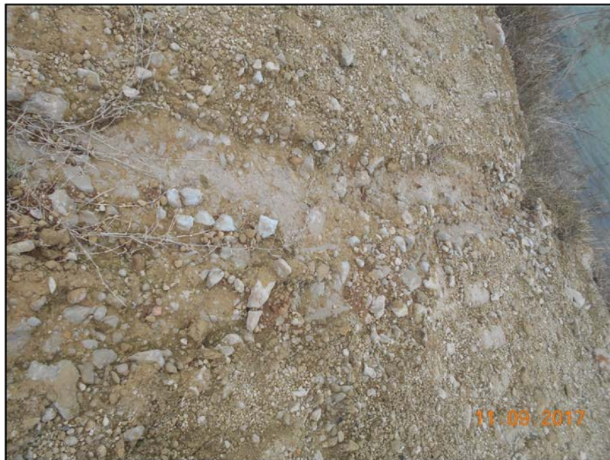
Photograph P-50 – Taken November 9, 2017 by David E. Nielson Landfill Cell 2B: Looking down at inside slope of landfill berm. Close up view of stabilized material that has stopped apparent erosion.
