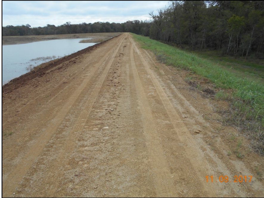
Photograph P-51 – Taken November 9, 2017 by David E. Nielson Landfill Cell 2B: Looking east along crest of the southern berm.
