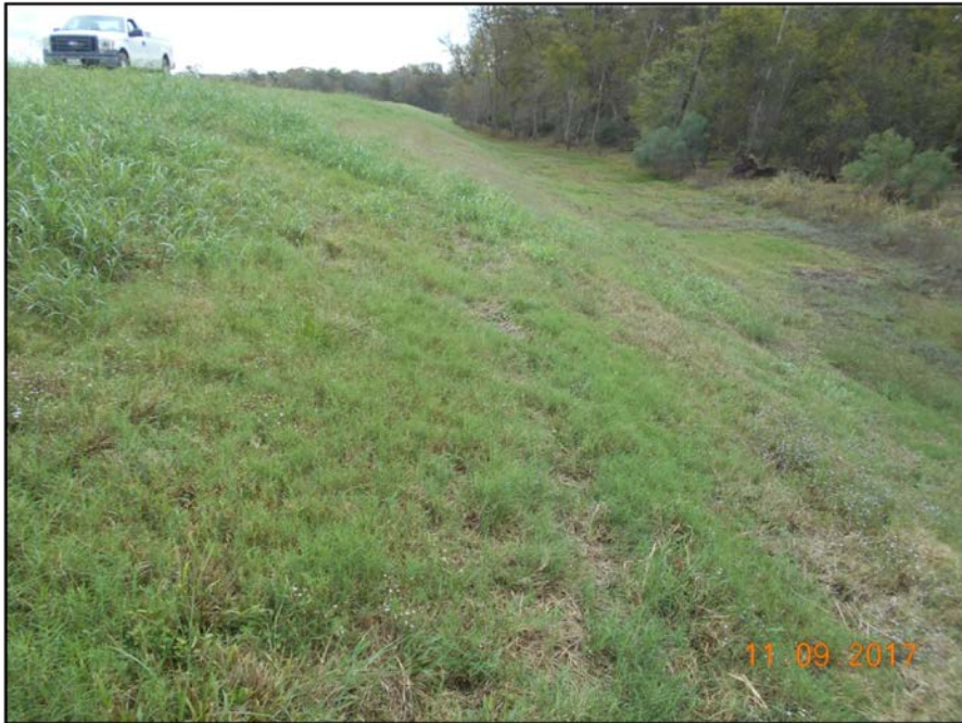
Photograph P-52 – Taken November 9, 2017 by David E. Nielson Landfill Cell 2B: Looking east along outside slope of southern berm.
