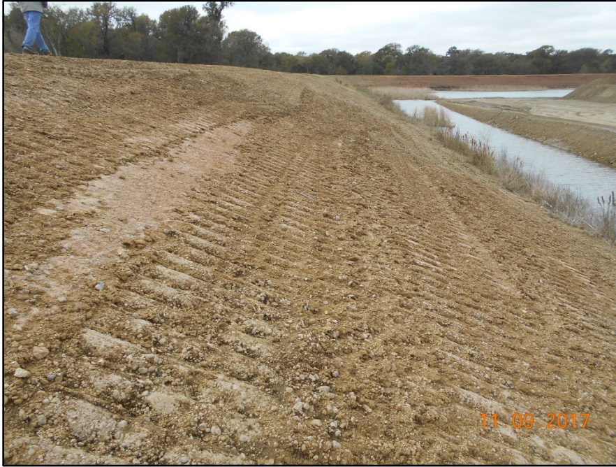
Photograph P-43 – Taken November 9, 2017 by David E. Nielson Landfill Cell 2B: Looking south along the inside slope of the eastern landfill berm.
