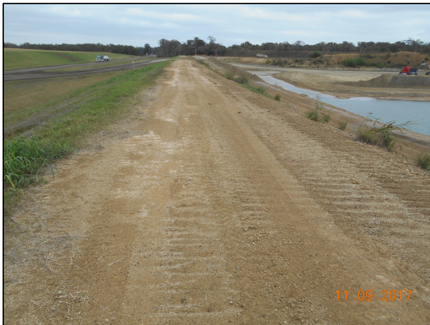
Photograph P-36 – Taken November 9, 2017 by David E. Nielson Landfill Cell 2B: Looking north along crest of western berm.
