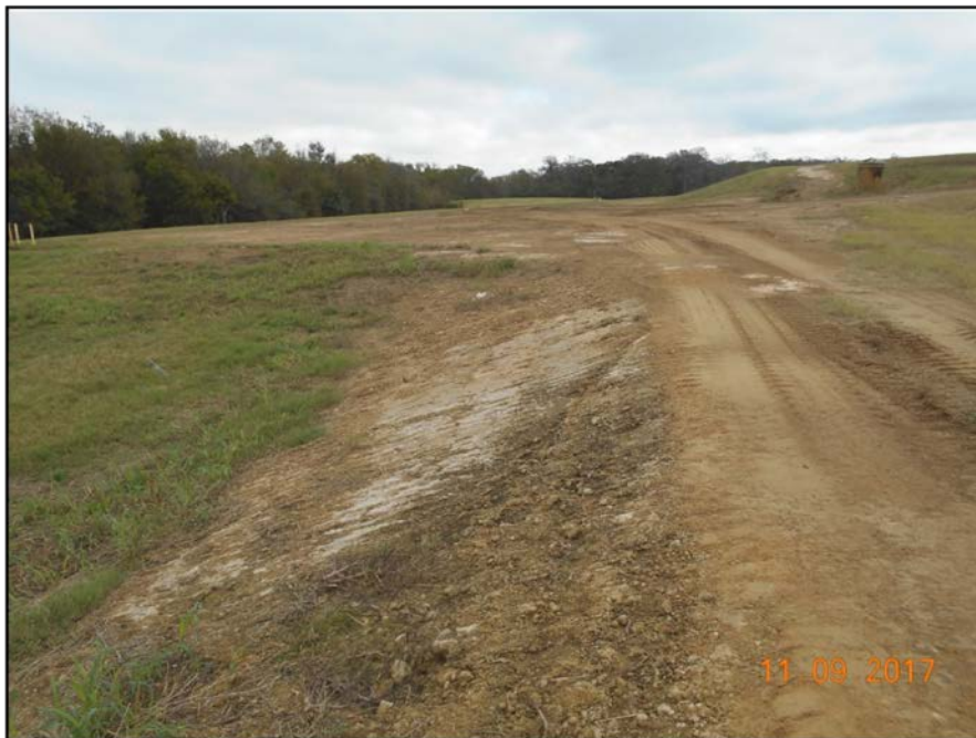
Photograph P-33 – Taken November 9, 2017 by David E. Nielson Landfill Cell 1C: Looking east along the outside slope of the northern berm.
