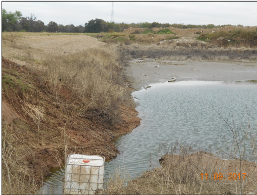
Photograph P-26 – Taken November 9, 2017 by David E. Nielson Landfill Cell 1C: Looking north along the inside slope of the western landfill berm at the incised storm water pond.
