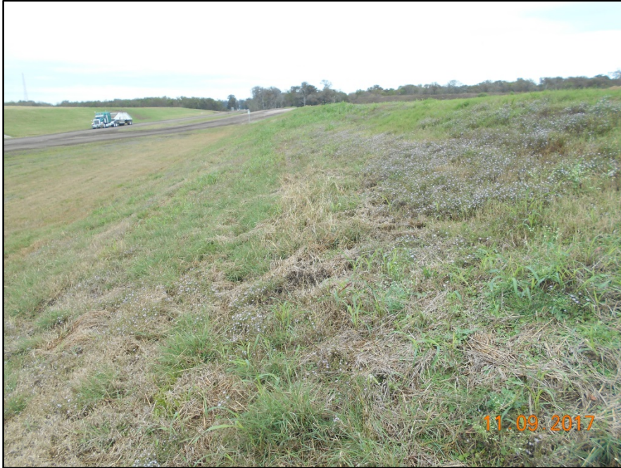
Photograph P-37 – Taken November 9, 2017 by David E. Nielson Landfill Cell 2B: Looking north along outside slope of western berm. Note good vegetation cover and uniform slope.
