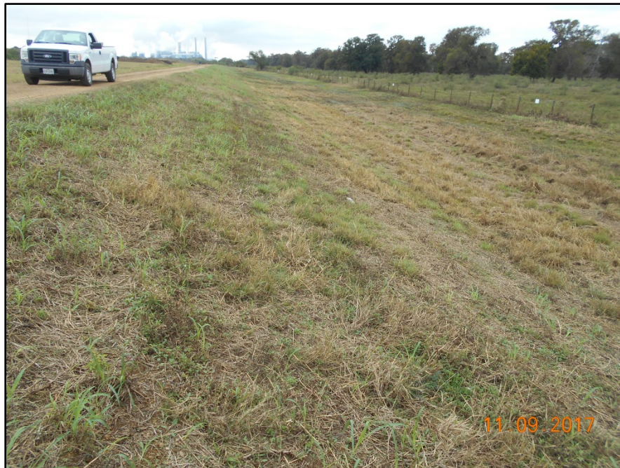
Photograph P-31 – Taken November 9, 2017 by David E. Nielson Landfill Cell 1C: Looking south along the outside slope of the western berm. Note good vegetation control.
