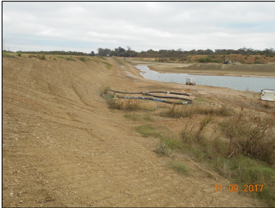
Photograph P-35 – Taken November 9, 2017 by David E. Nielson Landfill Cell 2B: Looking north along the inside slope of the western berm at the area where a mobile pump is placed to remove storm water collected in incised storm water pond located within the cell. Note the slope has been regraded with stabilized material to reduce future erosion. See Photograph 50.
