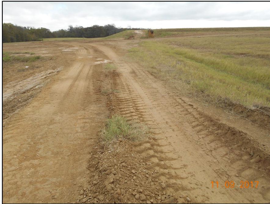
Photograph P-32 – Taken November 9, 2017 by David E. Nielson Landfill Cell 1C: Looking east along the crest of slope of the northern berm.
