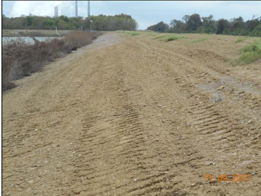
Photograph P-8 – Taken November 9, 2017 by David E. Nielson Landfill Cell 3: Looking south along inside slope of western berm of landfill cell in vicinity of incised storm water pond. Note this area that does not support vegetation is surfaced with stabilized material to control erosion. Also see Photograph 50.
