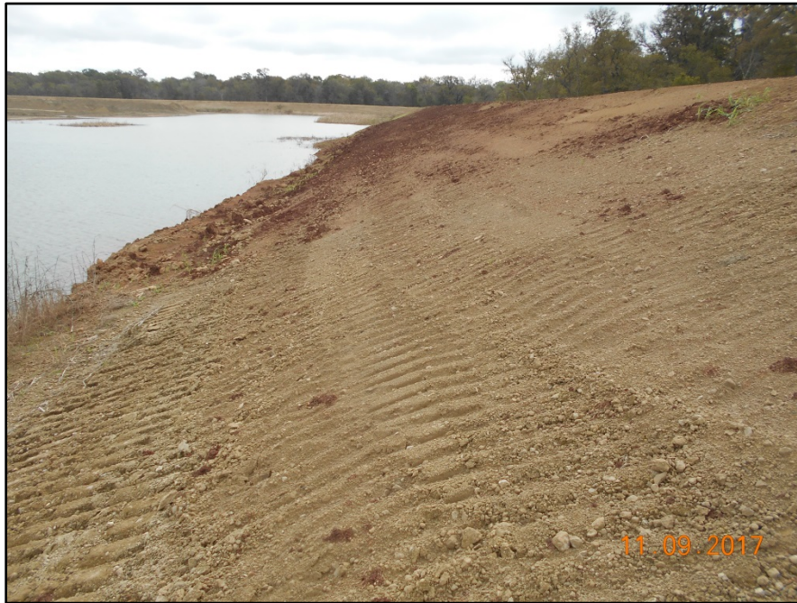
Photograph P-49 – Taken November 9, 2017 by David E. Nielson Landfill Cell 2B: Looking east along inside slope of southern berm.
