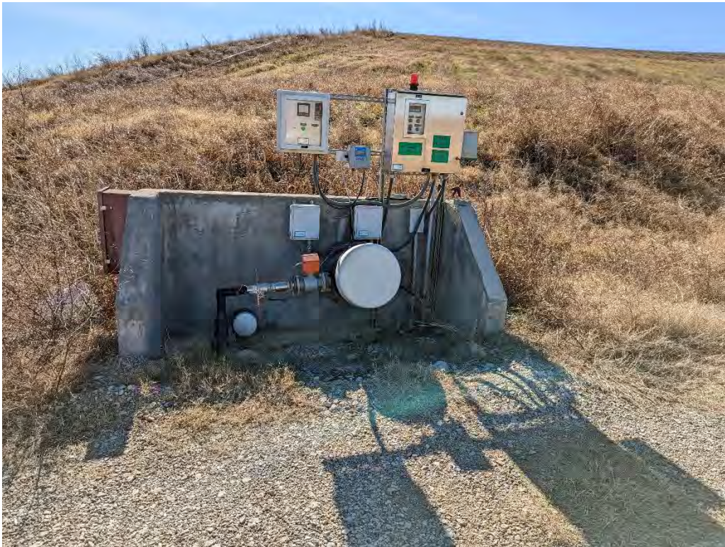
Photo 8. Typical Leachate Collection and Monitoring System
