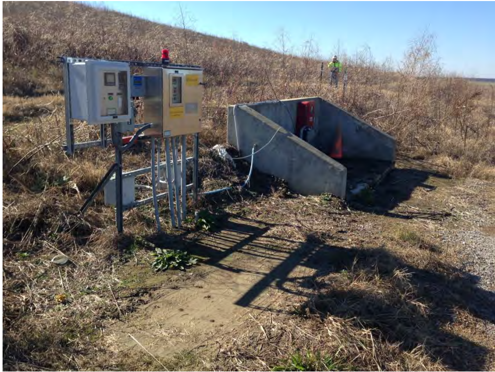
Photo 11: Typical leachate pumping system, Cell 1
