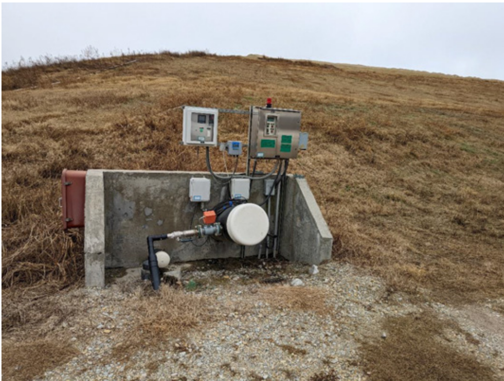
Photo 8. Typical leachate collection and monitoring system (Cell 3).
