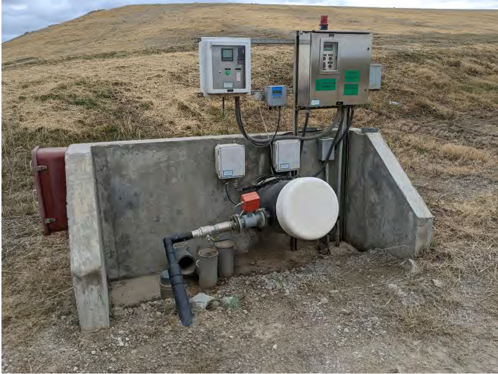
Photo 5. Typical Leachate Collection System monitoring and pumping system
