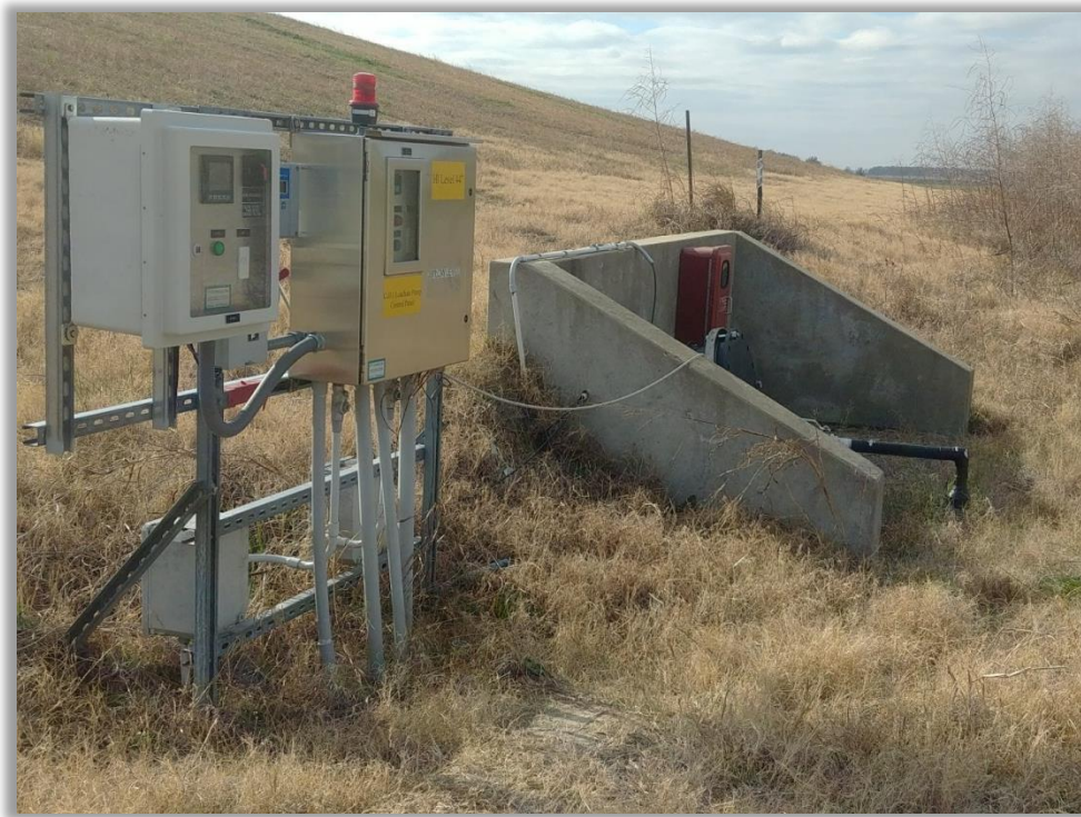
Photo 8: Cell 1 leachate pumping system.
