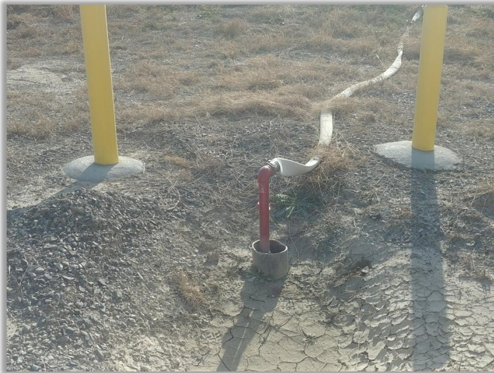
Photo 14: Dust control hydrant north side of Cell 3.
