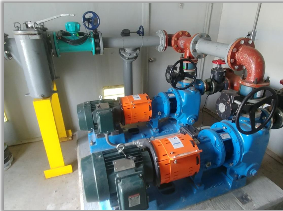
Photo 12: Leachate transfer station pumps.
