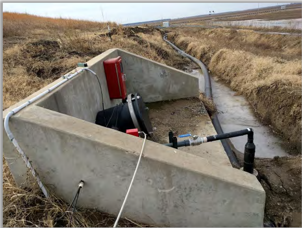
Photo 8: Cell 1 leachate pumping system. Note construction of forcemain to leachate storage pond.
