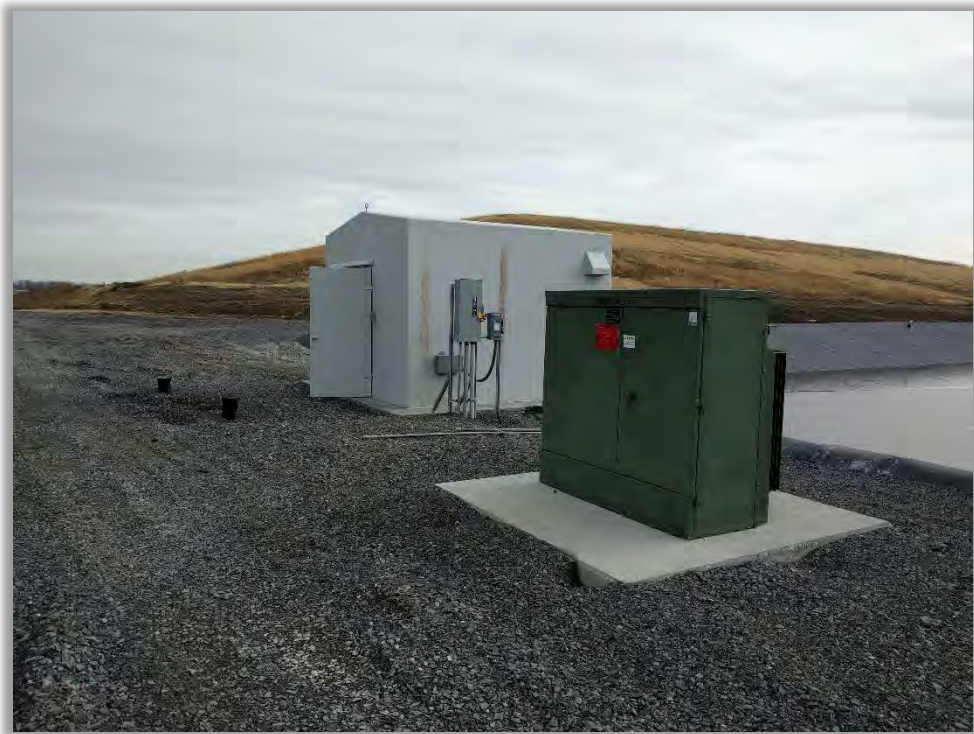
Photo 14: Leachate pump station.
