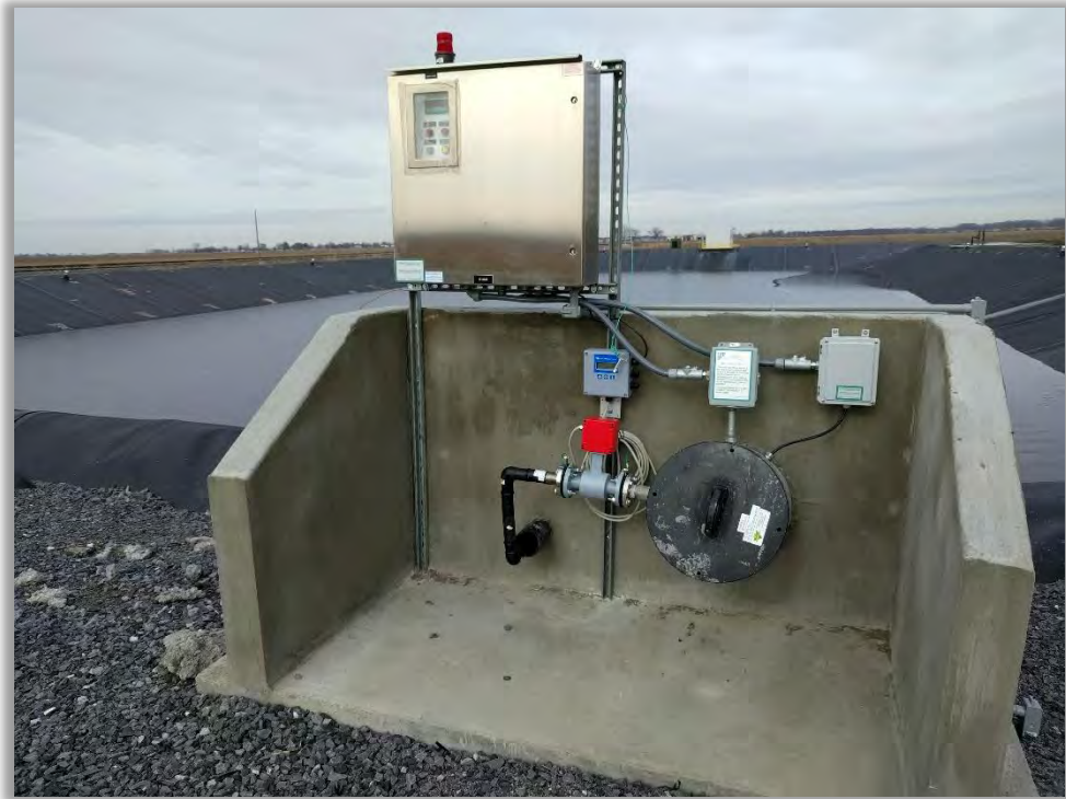
Photo 13: Leachate storage pond leak detection system pumping system.
