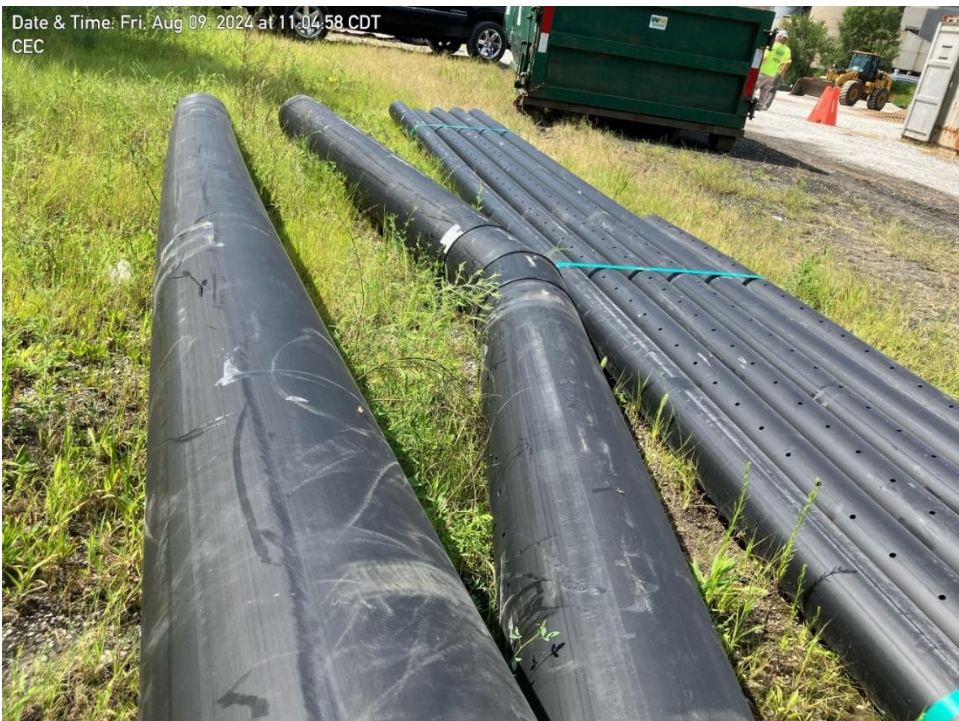
Photo 2: Perforations on sump pipe are aligned with the top of the pipe once it will be placed in the bypass basin.
