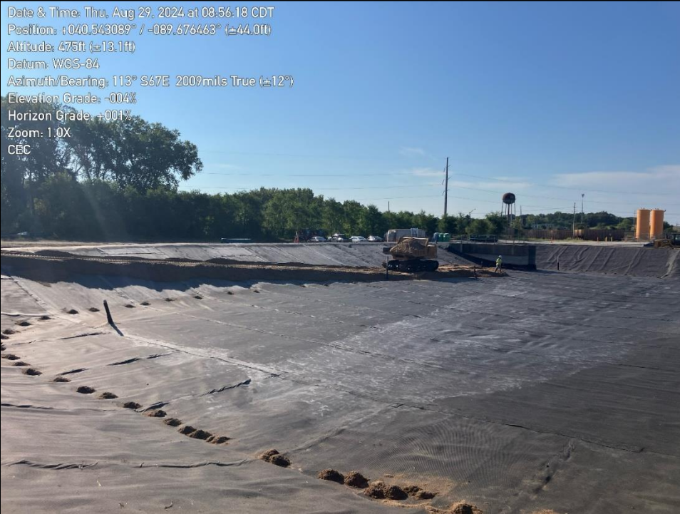
Photo 1: shows sand drainage layer being placed on the ramp into the basin.
