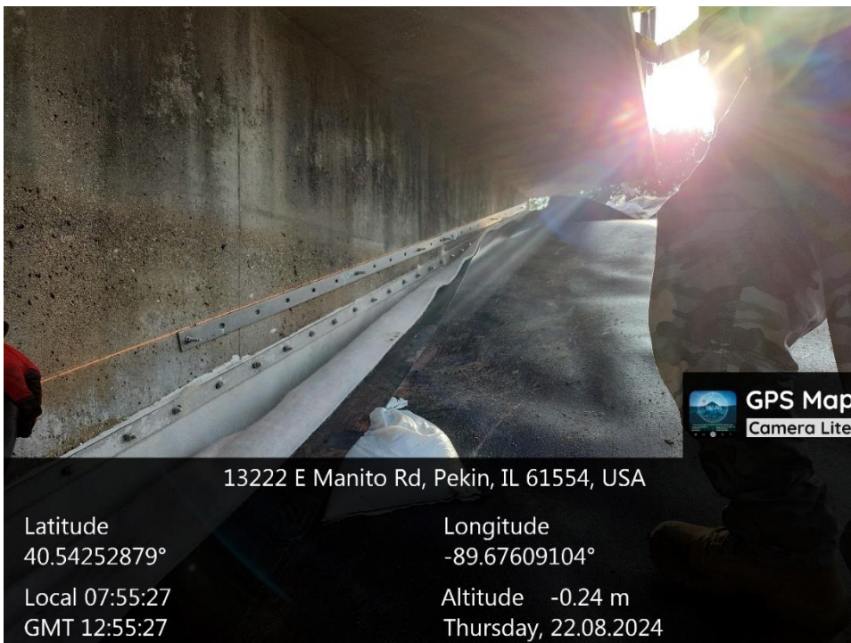
Photo 1: CAAWS crew installing bracing along the southeast concrete structure to secure the GCL and geomembrane to the structure.
