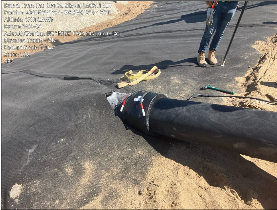
Photo 1: shows electro coupler on the 12" riser pipe.
