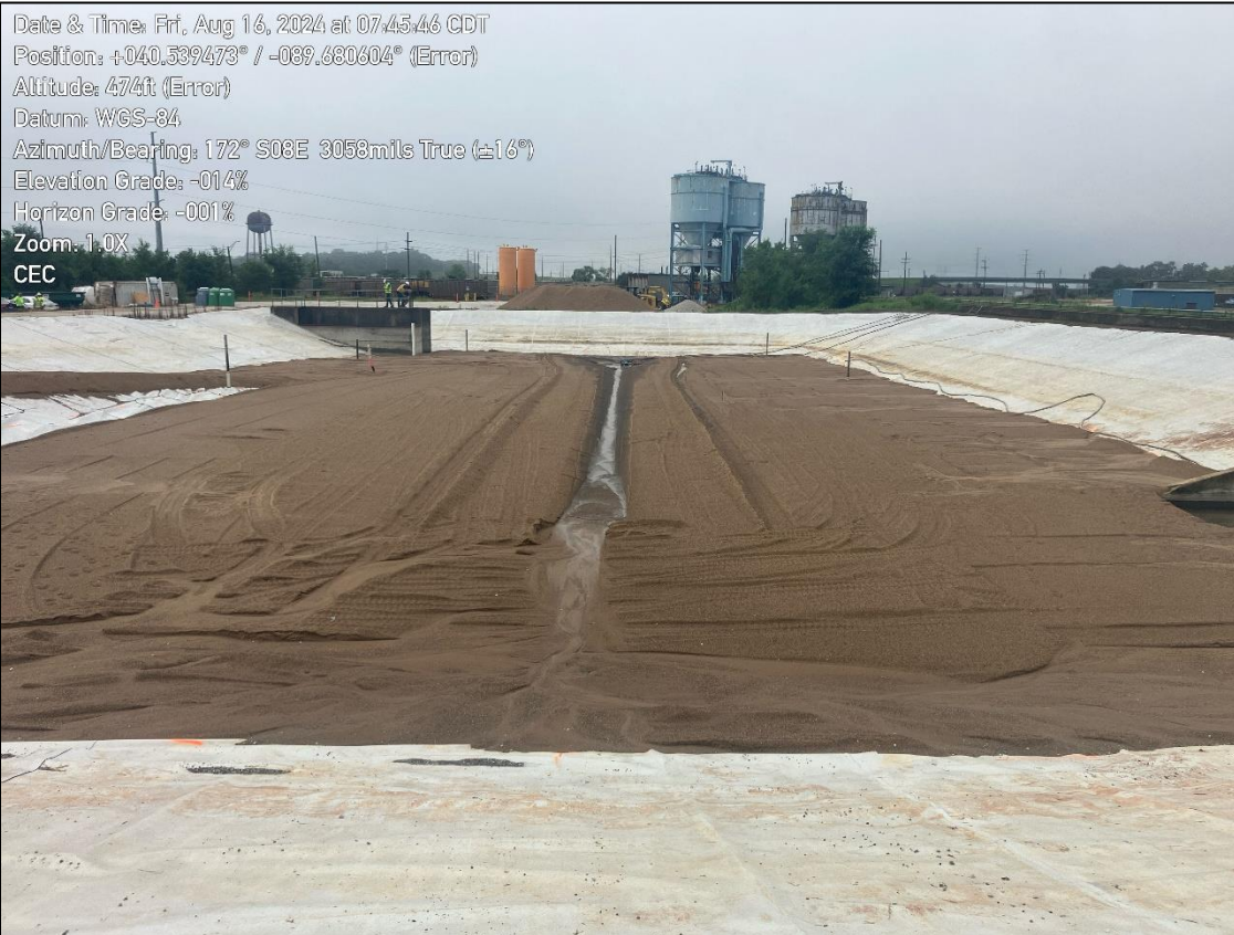
Photo 1: Structural fill after rain event.
