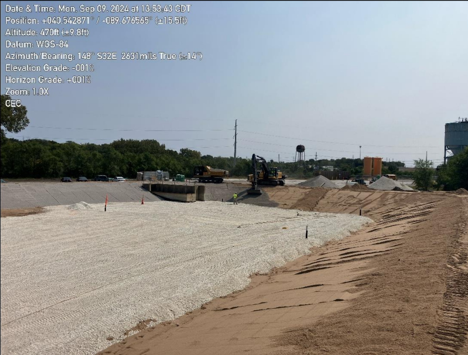
Photo 1: shows completed sand filter layer along slopes and rip rap bedding layer being placed.
