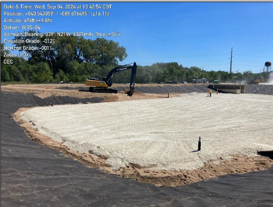
Photo 2: shows completed protective warning layer and placement of sand filter along slopes.
