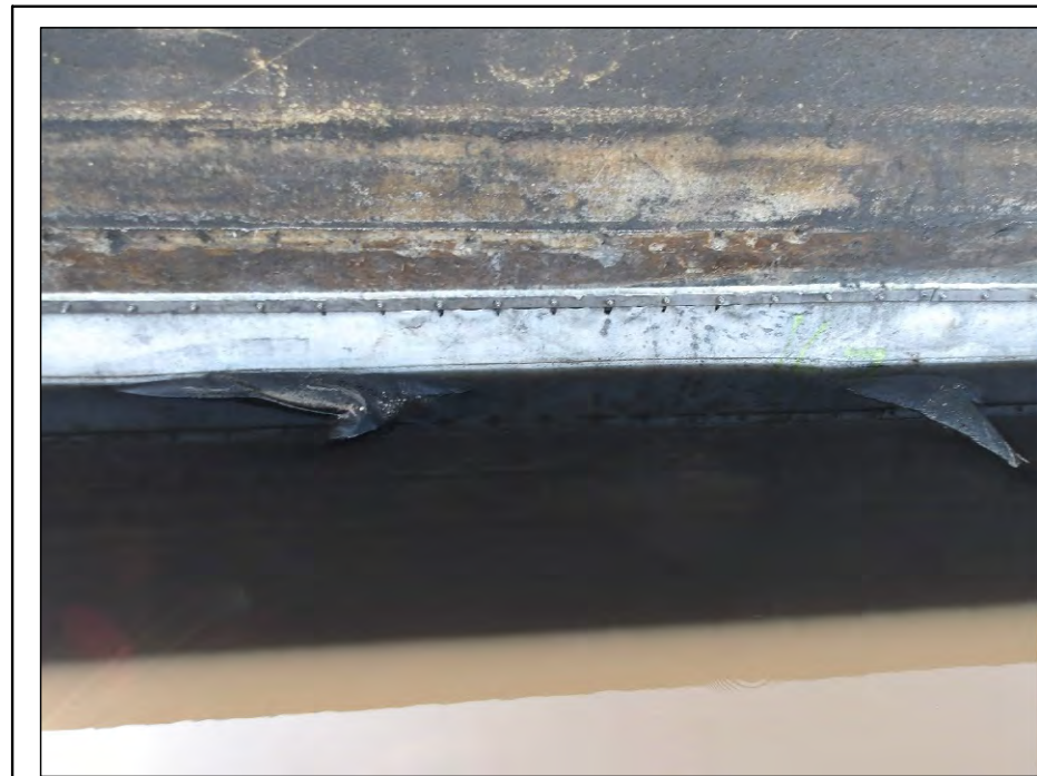
A BATTEN CONNECTION TO BE REMOVED
