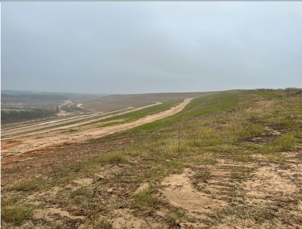
Photograph P-13: View looking southeast across recently installed final cover system in Area 1.
