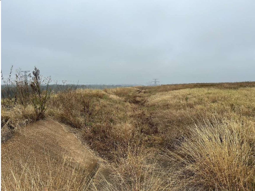
Photograph P-4: View looking north at the drainage ditch located along the perimeter of the top of the landfill. This ditch drains to the concrete outfall structure shown in Photograph P-3. The ditch appeared to flow well, without significant rutting or standing water.
