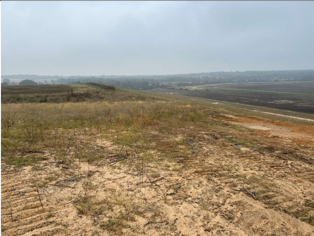
Photograph P-12: View looking north across installed clay cover system in Area 3.
