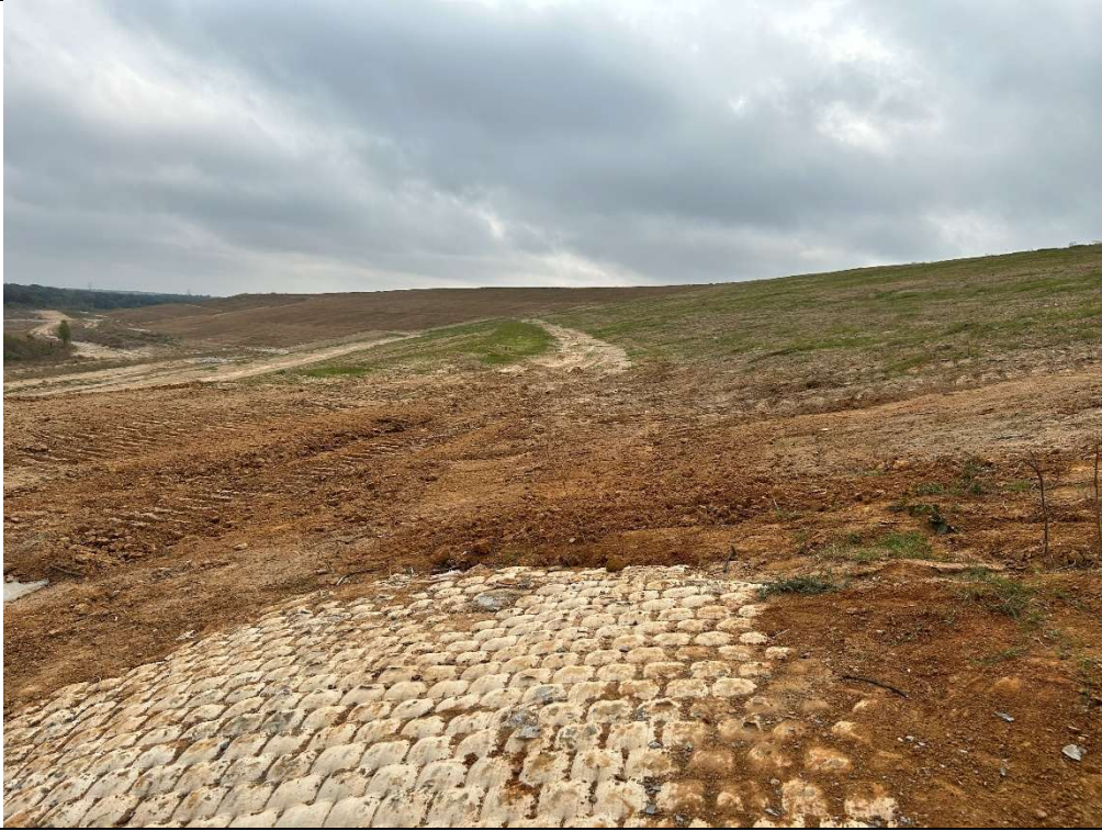
Photograph P-11: View looking east of newly installed final cover system in Area 4. Revegetation is in progress.
