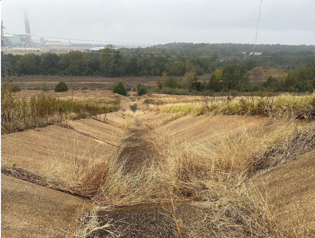
Photograph P-3: View looking west-southwest down concrete outfall in Area 5. A stormwater ditch located along the perimeter of the top of the landfill drains to this concrete outfall (also in Photograph P-4).
