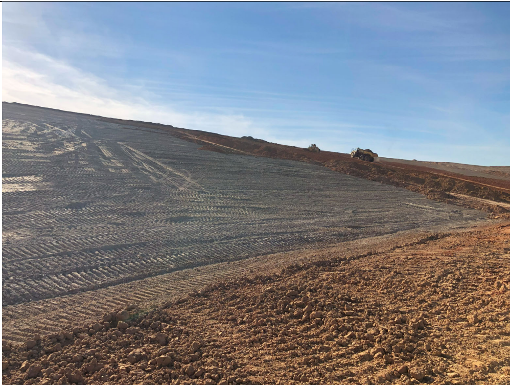
Photograph P-11: View looking west of graded CCR waste in Area 4. A final cover system will be installed on this portion of the landfill.
