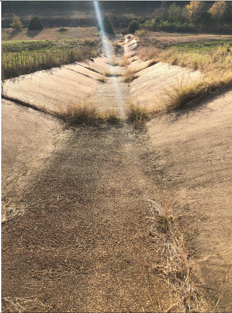
Photograph P-3: View looking west-southwest down concrete outfall in Area 5. A stormwater ditch located along the perimeter of the top of the landfill drains to this concrete outfall (also in Photograph P-4).
