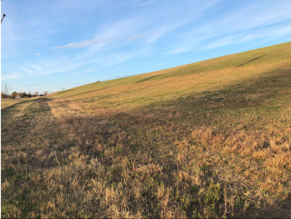
Photograph P-6: View looking north up the side slope of Area 2. The terraced slope is well vegetated with no visible sloughing or erosional issues.
