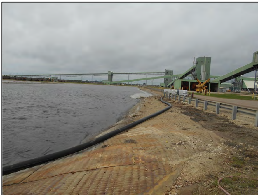
Photograph P-3 – Taken November 11, 2015 by David E. Nielson Pond K: Looking west along the northern bank, which is incised. This verifies that the Federal CCR Rule regarding inspections does not apply to Pond K.
