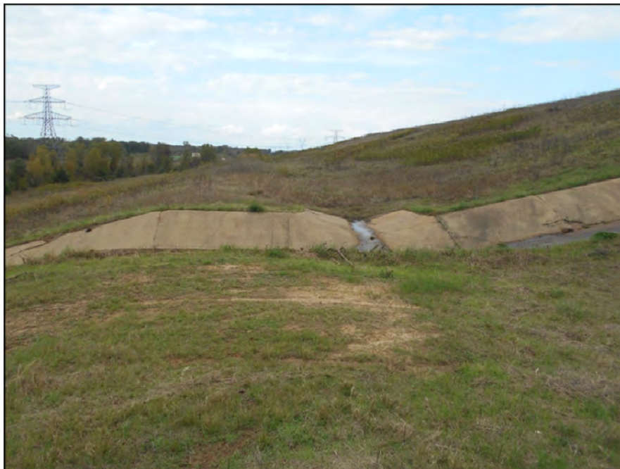
Photograph P-61 – Taken November 11, 2015 by David E. Nielson Landfill Area 5: Looking northwest along the mid-slope bench. Note good slope uniformity and good vegetation cover.
