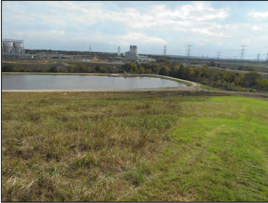
Photograph P-72 – Taken November 11, 2015 by David E. Nielson Landfill Area 9: Looking southeast and down slope to where landfill drains into Pond 002. Note good vegetation and lack of erosion.
