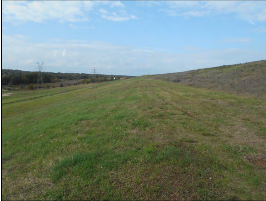
Photograph P-68 – Taken November 11, 2015 by David E. Nielson Landfill Area 9: Looking northwest along the mid-slope bench in the capped landfill slope. Note good vegetation cover and lack of erosion of slope.
