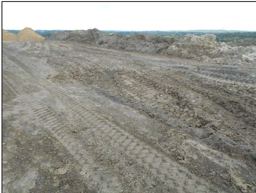
Photograph P-83 – Taken November 11, 2015 by David E. Nielson Landfill Area 8 (uncapped area): Looking east at crest of temporary slope shown in Photographs P-81 and P-82. Note uncapped placement of CCR material to prevent further erosion of temporary slope face.
