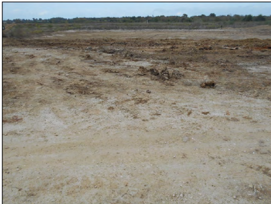
Photograph P-87 – Taken November 11, 2015 by David E. Nielson Landfill Area 20 (area under construction): Looking northwest at area that has been partially cleared and grubbed in preparation for placement of clay liner for Area 20.
