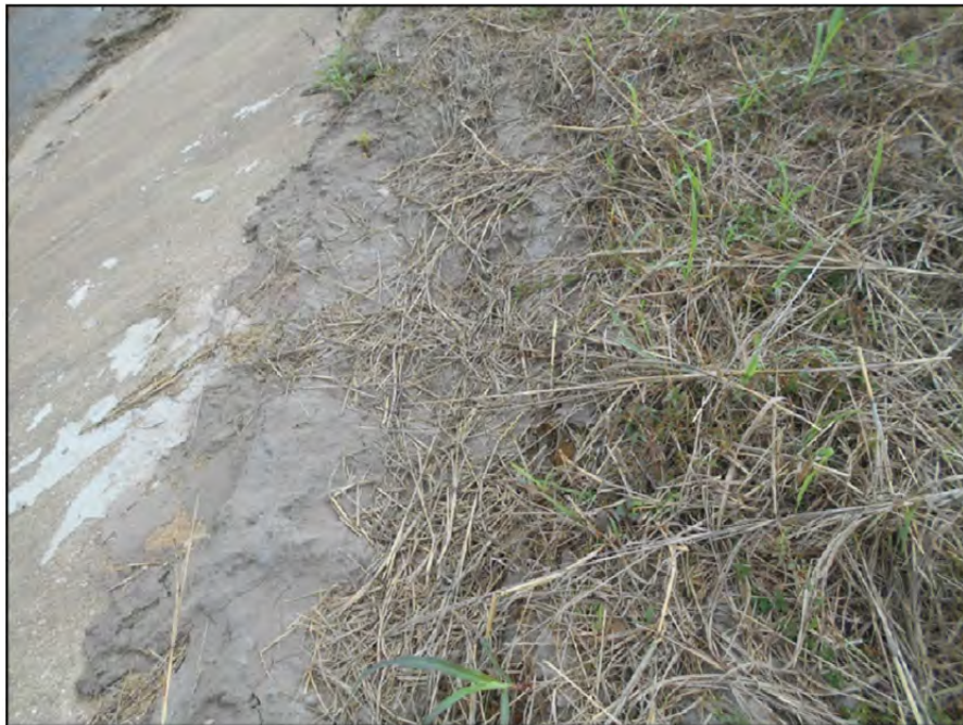
Photograph P-57 – Taken November 11, 2015 by David E. Nielson Landfill Area 1: Looking at grouted repair of an area of stormwater concrete lined rundown channel that was previously undermined.
