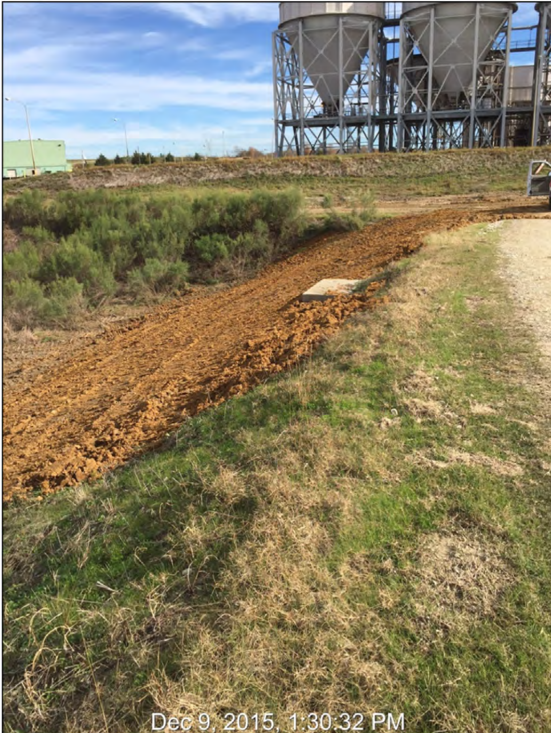
Photograph P-22 – Taken December 9, 2015 by NRG Pond ST-18: Looking east at outside slope of northern edge of pond. Note the steep dike section depicted in Photographs P-20 and P-21 has been corrected with the addition of compacted fill. Grass cover should be established over new fill.
