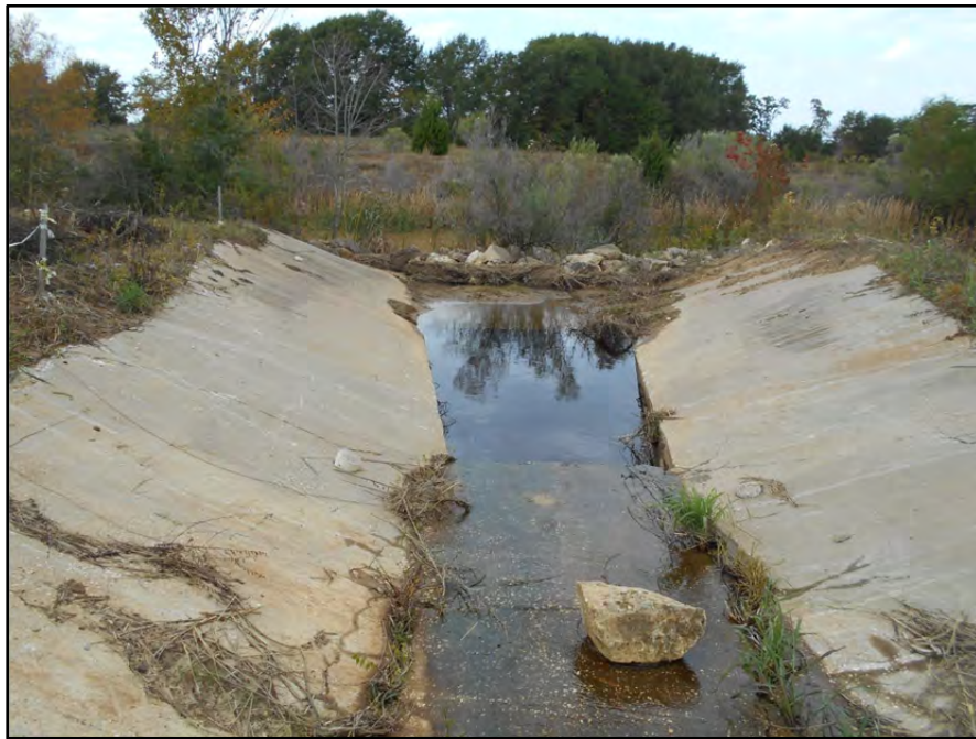
Photograph P-56 – Taken November 11, 2015 by David E. Nielson Landfill Area 1: Looking northwest at stormwater rundown channel discharge into perimeter ditch. Note energy dissipation pit and riprap at mouth of discharge. Also note vegetation in perimeter ditch, which indicates sufficient velocity control of stormwater.
