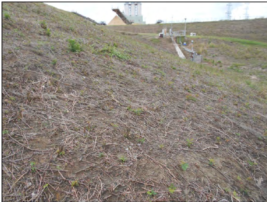
Photograph P-24 – Taken November 11, 2015 by David E. Nielson Pond ST-18: Looking south at outside slope western dike. Evidence of recent vegetation cutting was observed. Grass should be reestablished to reduce the risk of erosion of the outside slope.
