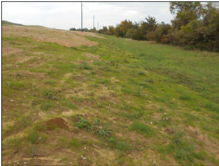
Photograph P-50 – Taken November 11, 2015 by David E. Nielson Pond 002: Looking east along the outside slope and toe of slope of the southern dike.
