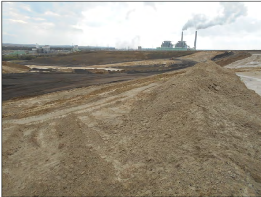
Photograph P-80 – Taken November 11, 2015 by David E. Nielson Landfill Area 11(uncapped area): Looking southwest at active disposal area.
