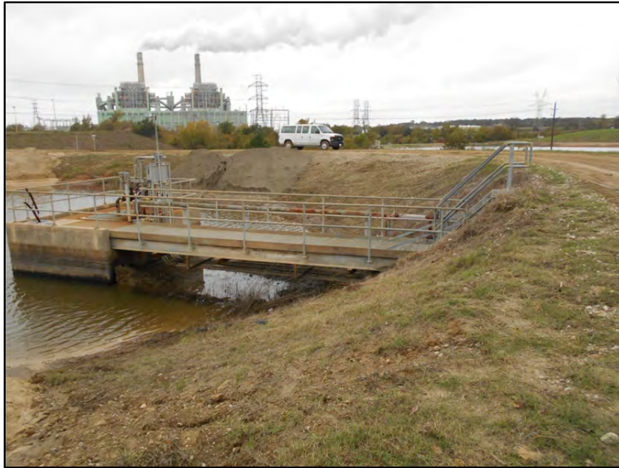
Photograph P-19 – Taken November 11, 2015 by David E. Nielson Pond ST-18: Looking west at inside slope of north dike of pond and outlet structure.
