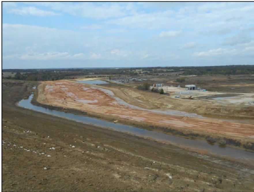
Photograph P-89 – Taken November 11, 2015 by David E. Nielson Landfill Area 13 (area under construction): Looking north at area that has been cleared and grubbed, with partial placement of clay liner (reddish brown material).
