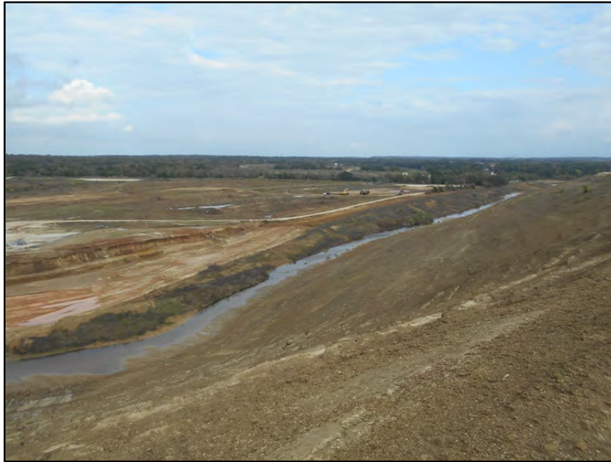
Photograph P-88 – Taken November 11, 2015 by David E. Nielson Landfill Area 20 in background and landfill Area 19 in foreground: Looking northeast from top of landfill Area 7. Note Area 20 ongoing construction tasks to clear and grub in preparation for placement of clay liner, while Area 19 has been cleared and grubbed except along perimeter interceptor ditch, which will be relocated. Some reddish brown clay liner has been placed in Area 19.
