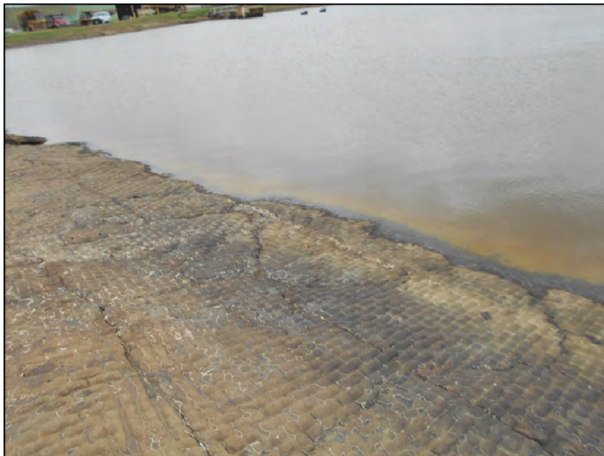
Photograph P-7 – Taken November 11, 2015 by David E. Nielson Pond E: Looking west at the fabriform erosion protection blanket on the southern bank at the pipe discharge. Although cracks are present, it is functional in preventing erosion.
