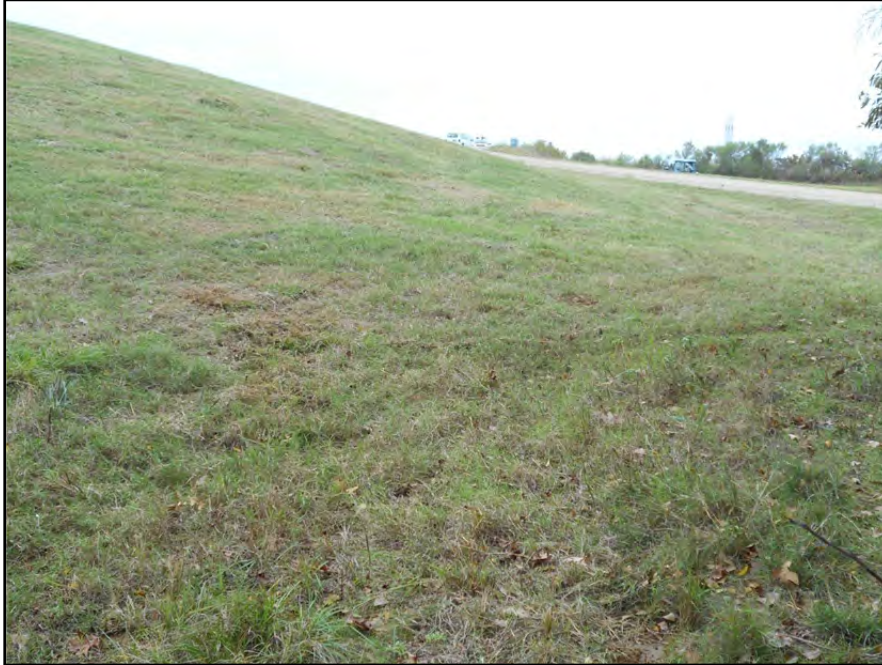
Photograph P-42 – Taken November 11, 2015 by David E. Nielson Secondary E Pond: Looking south along the outside slope of the western dike and the dike toe. Note good grass vegetation in most areas. Note good slope and alignment.
