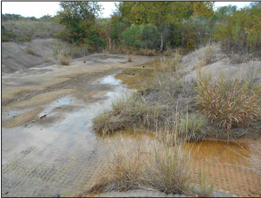
Photograph P-66 – Taken November 11, 2015 by David E. Nielson Landfill Area 5: Looking northwest at perimeter ditch upstream from discharge of concrete lined stormwater runoff channel. Note significant vegetation in upstream ditch, which should be removed before additional stormwater flows from upstream landfill areas are diverted into this ditch.
