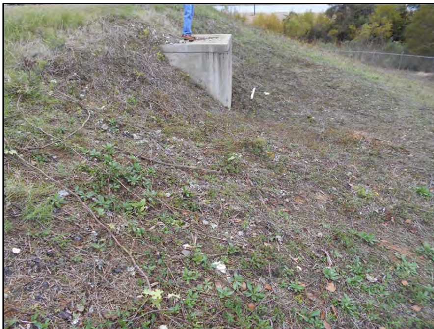
Photograph P-20 – Taken November 11, 2015 by David E. Nielson Pond ST-18: Looking west at outside slope of northern edge of pond. Note the steep dike section in the vicinity of the outlet structure manhole. This dike is steeper than typical. Additional fill should be placed and compacted to lessen the steepness of the slope and increase the dike stability. No evidence of dike instability was noted.
