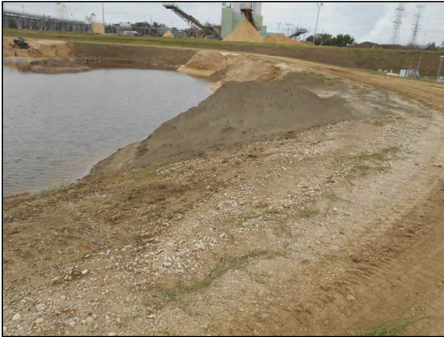
Photograph P-23 – Taken November 11, 2015 by David E. Nielson Pond ST-18: Looking south at inside slope of western dike.
