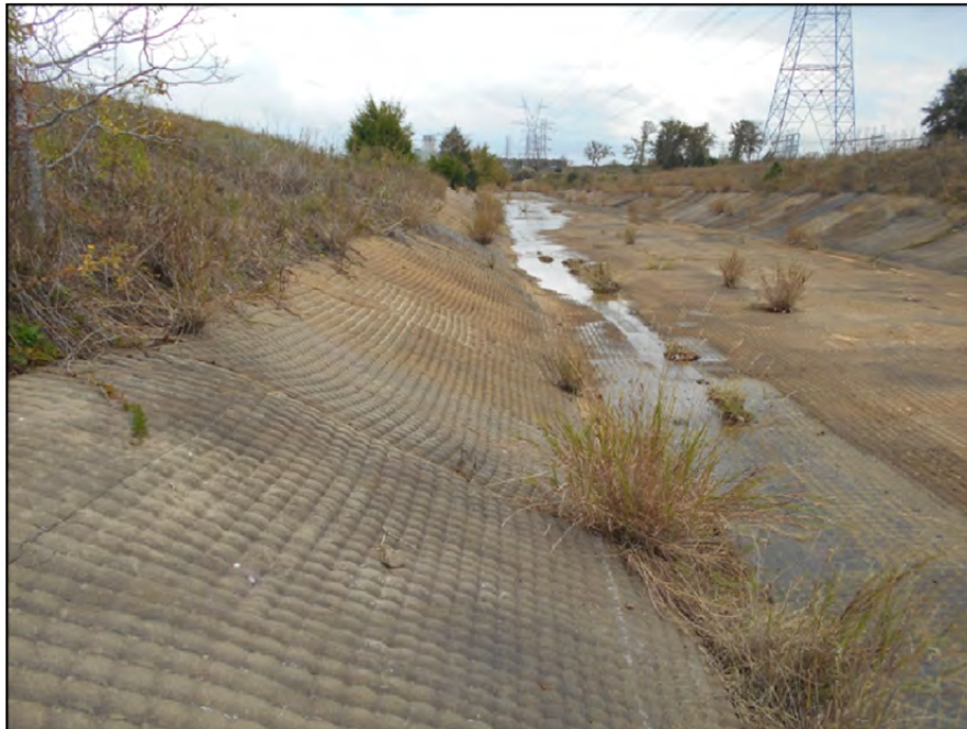
Photograph P-67 – Taken November 11, 2015 by David E. Nielson Landfill Area 5: Looking southeast along the perimeter ditch downstream from the discharge of concrete lined stormwater runoff channel. Note good condition of fabric form concrete lining.
