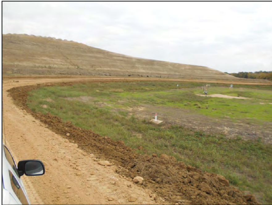
Photograph P-78 – Taken November 11, 2015 by David E. Nielson Landfill Area 11(uncapped area): Looking northeast at an uncapped CCR material slope that will be capped when Area 11 is capped. Note eroded material is intercepted in perimeter ditch that drains to Pond 002.
