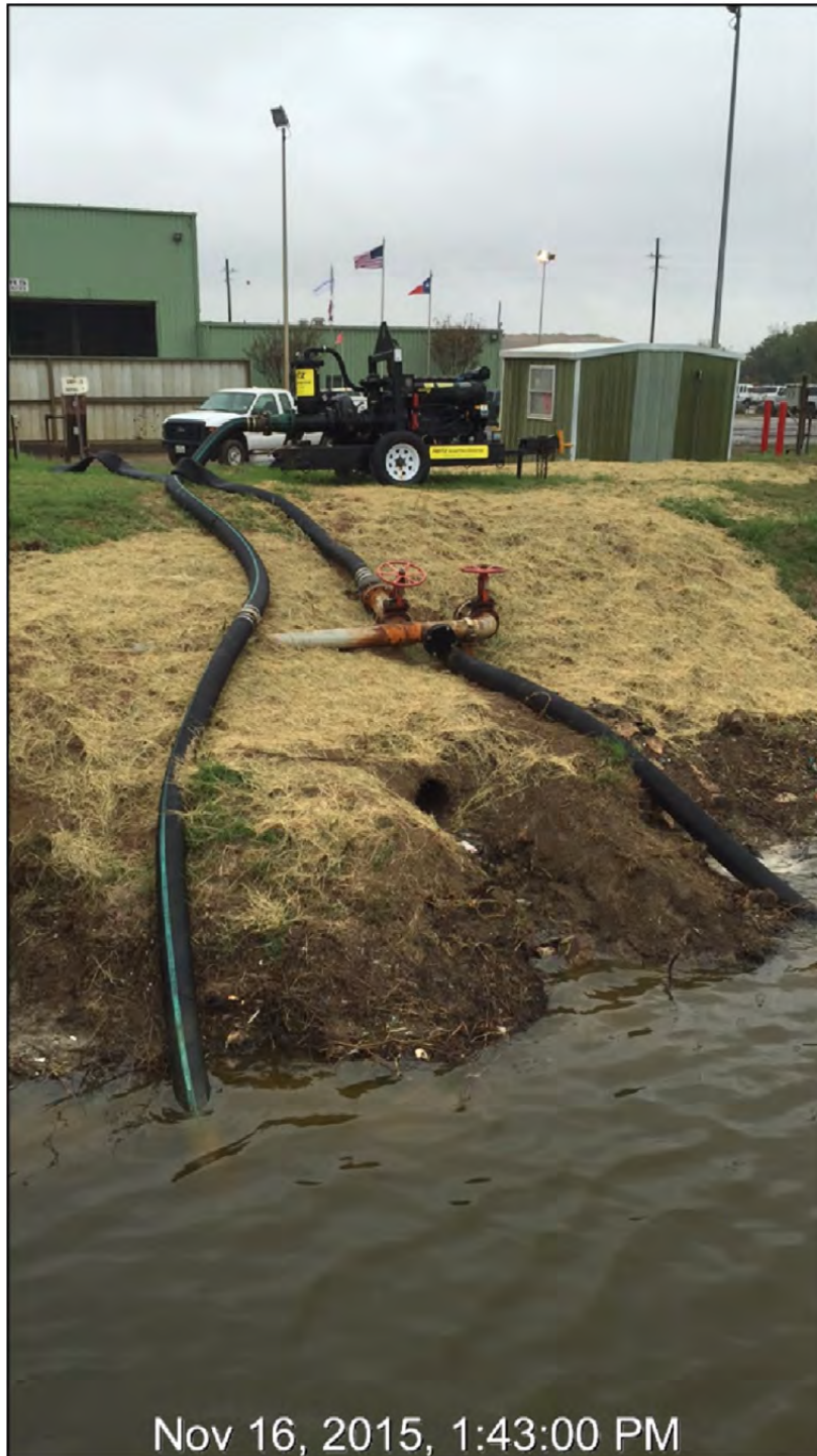
Photograph P-15 – Taken November 16, 2015 by NRG Pond E: Looking north at the inside slope of the north dike (the area of Photographs P-13 and P-14). Note pipe discharge has been exposed. The valve and hose area has been cleaned up and the area has been seeded.
