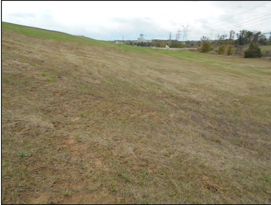
Photograph P-64 – Taken November 11, 2015 by David E. Nielson Landfill Area 5: Looking southeast along the toe of side slope of capped landfill. Note slope uniformity and absence of erosion.
