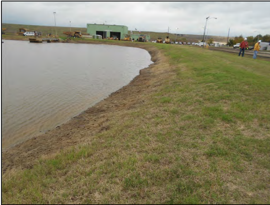
Photograph P-10 – Taken November 11, 2015 by David E. Nielson Pond E: Looking north at the inside slope of the eastern dike. Although, some minor slope irregularity was noted, there was no evidence of structural instability observed.
