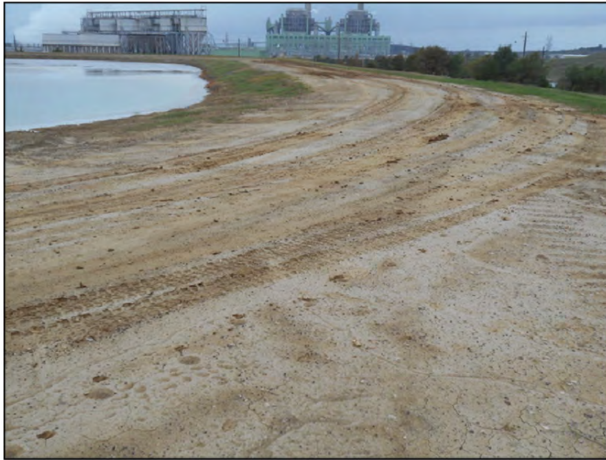
Photograph P-36 – Taken November 11, 2015 by David E. Nielson Secondary E Pond: Looking west at inside slope of the northern dike. Note traffic rutting of top of dike.
