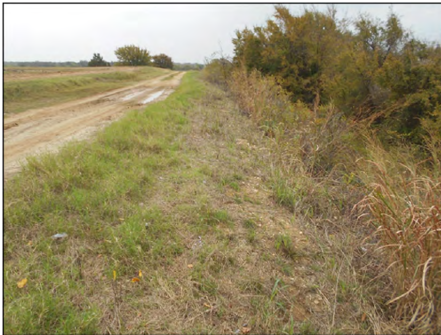
Photograph P-31 – Taken November 11, 2015 by David E. Nielson Secondary E Pond: Looking east at outside slope of southern dike. Note the rutting and ponded water in the roadway. Also note excessive vegetation a significant distance from pond. Given this distance, roots of woody vegetation have little impact on pond performance.
