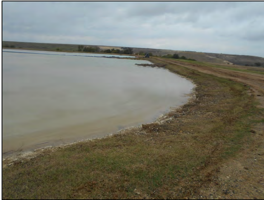
Photograph P-32 – Taken November 11, 2015 by David E. Nielson Secondary E Pond: Looking north along the inside slope of the eastern dike.
