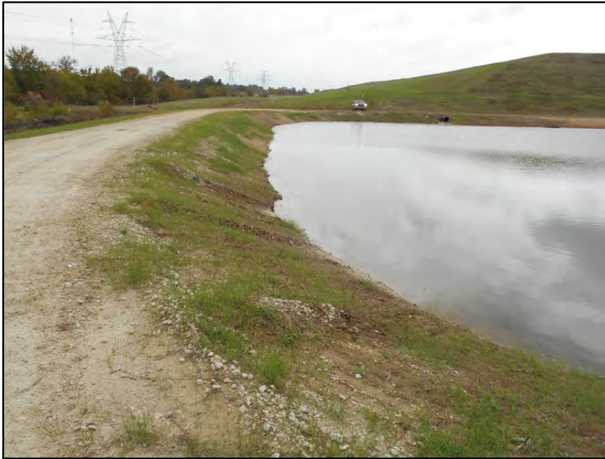
Photograph P-45 – Taken November 11, 2015 by David E. Nielson Pond 002: Looking north along the inside slope of the western dike.
