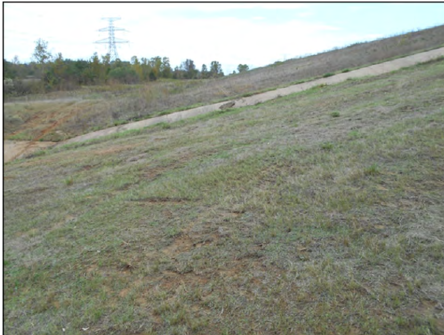
Photograph P-63 – Taken November 11, 2015 by David E. Nielson Landfill Area 5: Looking northwest at toe of side slope of capped landfill with concrete rundown channel. Note good vegetation cover, landfill slopes and absence of erosion.
