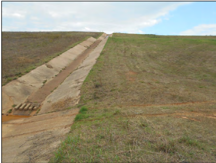
Photograph P-65 – Taken November 11, 2015 by David E. Nielson Landfill Area 5: Looking northeast at concrete lined stormwater rundown channel. Note generally good condition of the concrete lining, energy dissipation blocks and vegetation. Several minor areas of sparse grass are noted.
