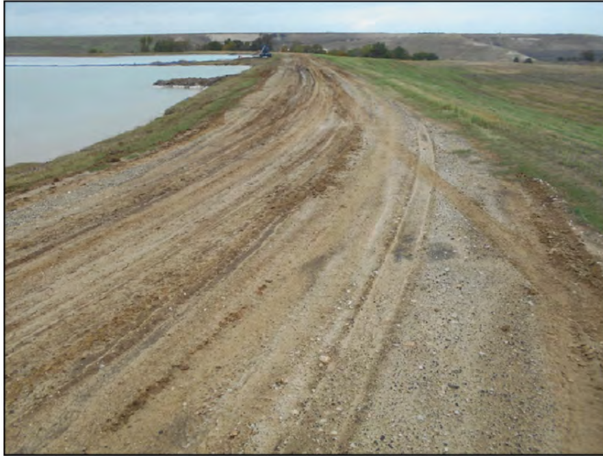
Photograph P-34 – Taken November 11, 2015 by David E. Nielson Secondary E Pond: Looking north along the eastern dike crest.
