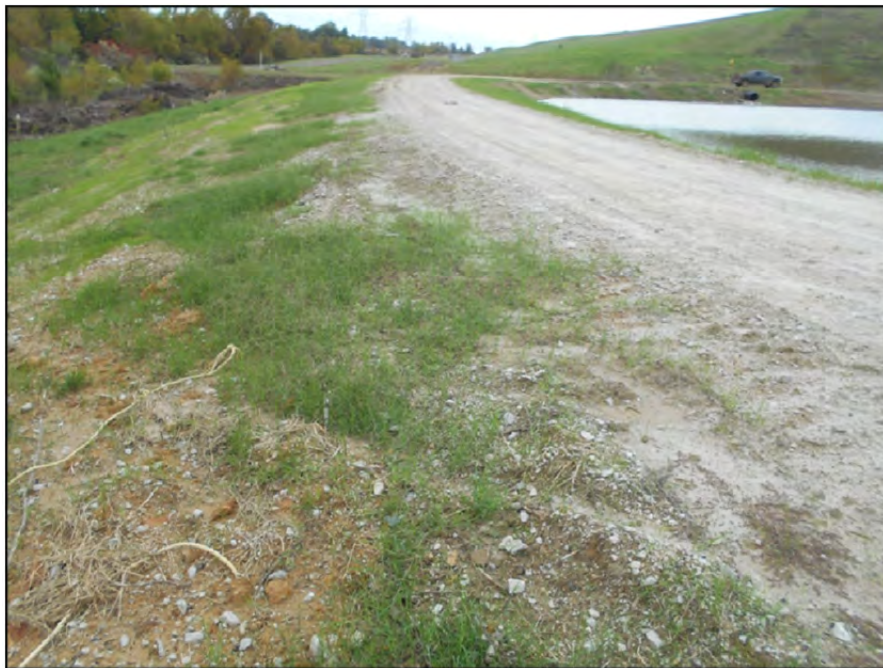
Photograph P-46 – Taken November 11, 2015 by David E. Nielson Pond 002: Looking north along the crest and outside slope of the western dike.
