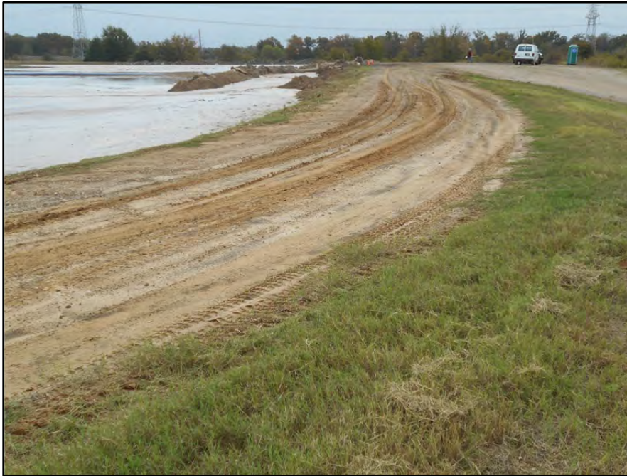
Photograph P-40 – Taken November 11, 2015 by David E. Nielson Secondary E Pond: Looking south at inside slope of the western dike.
