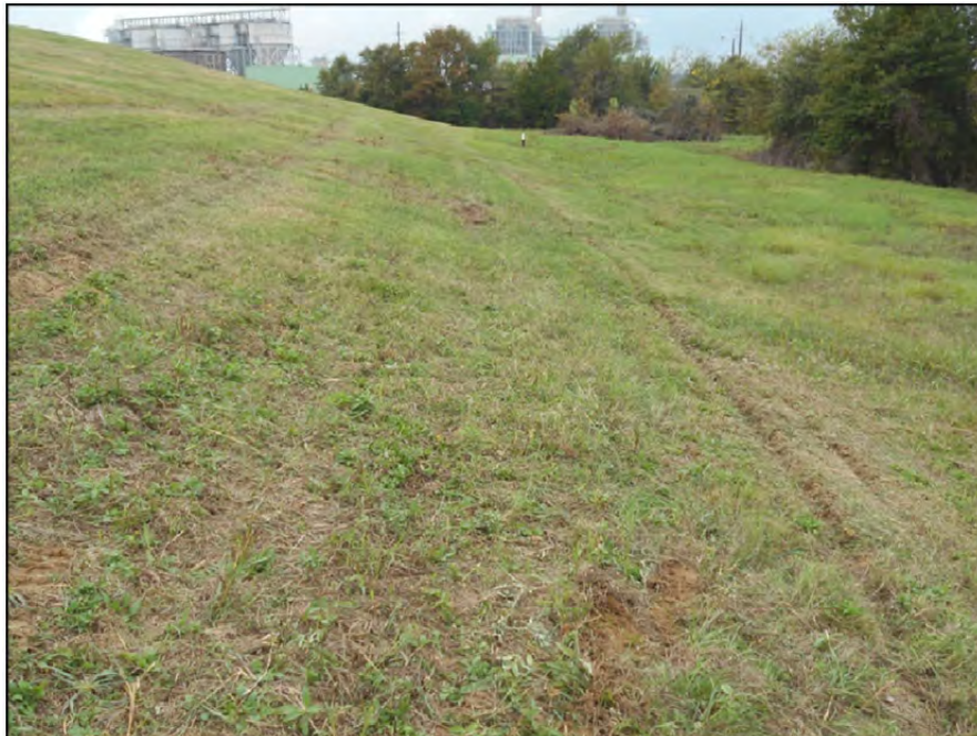
Photograph P-39 – Taken November 11, 2015 by David E. Nielson Secondary E Pond: Looking west along the outside slope and toe of slope of the northern dike. Note good grass vegetation in most areas. Note good slope and alignment.
