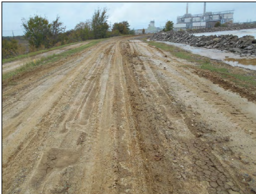
Photograph P-29 – Taken November 11, 2015 by David E. Nielson Secondary E Pond: Looking west along the southern dike crest and inside slope. Note rutting of dike crest.
