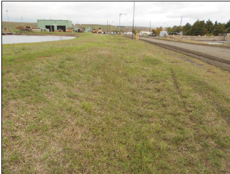
Photograph P-9 – Taken November 11, 2015 by David E. Nielson Pond E: Looking north at the outside slope of the eastern dike.
