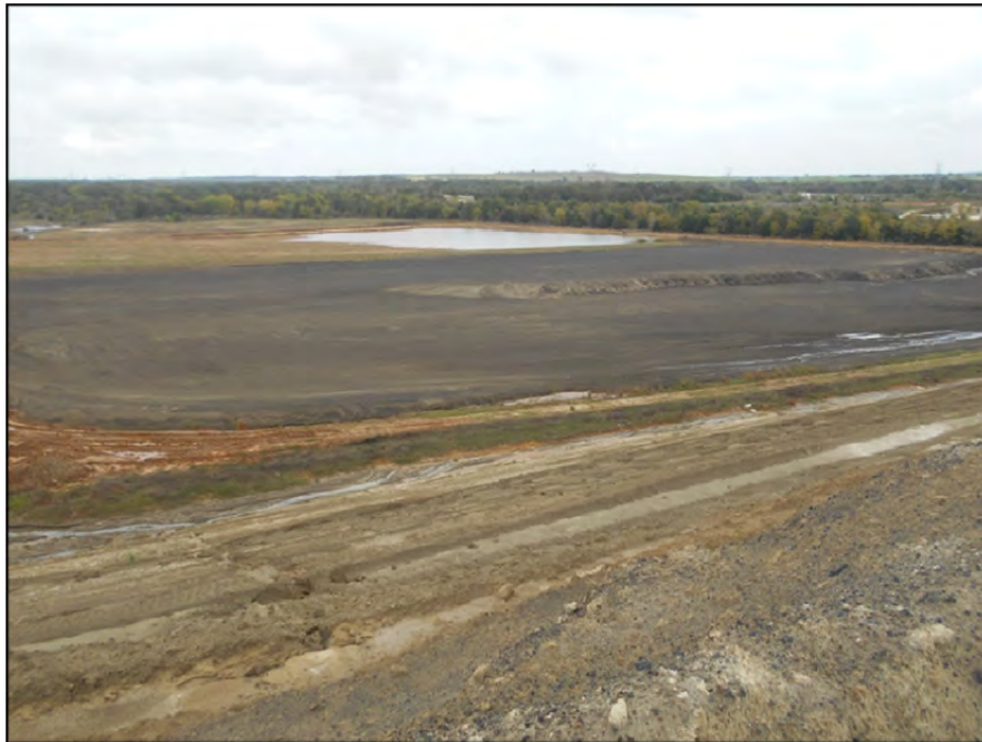
Photograph P-85 – Taken November 11, 2015 by David E. Nielson Landfill Area 12 (area under construction): Looking southeast from top of uncapped landfill at landfill Area 12. Note clay liner (reddish tan in background), protective layer over liner (gray material) and construction of new perimeter interceptor ditch in distant background, with interceptor ditch in foreground.
