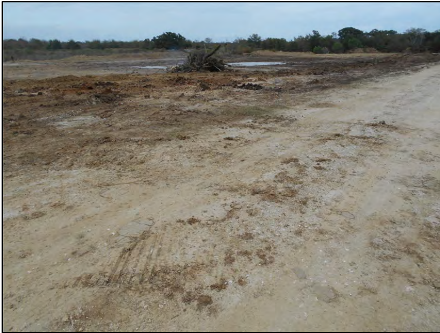
Photograph P-86 – Taken November 11, 2015 by David E. Nielson Landfill Area 20 (area under construction): Looking northeast at area that has been partially cleared and grubbed in preparation for placement of clay liner for landfill Area 20.
