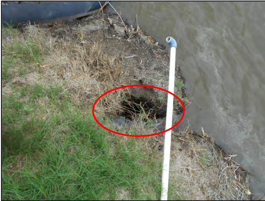
Photograph P-14 – Taken November 11, 2015 by David E. Nielson Pond E: Looking at the inside slope of the north dike where an erosional feature in slope appears to be a broken stormwater pipe discharging into pond.
