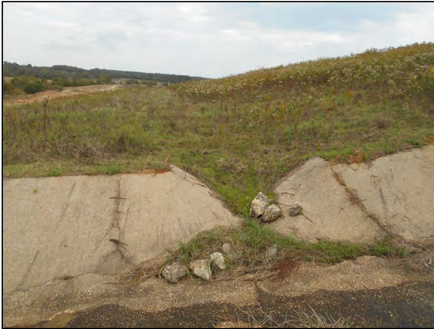
Photograph P-54 – Taken November 11, 2015 by David E. Nielson Landfill Area 1: Looking northeast at mid-slope bench and stormwater inlet into rundown channel. Note good vegetation on landfill cover (cap).
