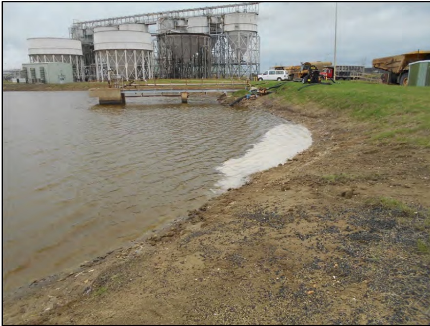
Photograph P-12 – Taken November 11, 2015 by David E. Nielson Pond E: Looking west at the inside slope of the north dike. Note the slope appears to be steeper than typical. The steep slope appears to be the result of excavations to remove collected solids from inside the pond.
