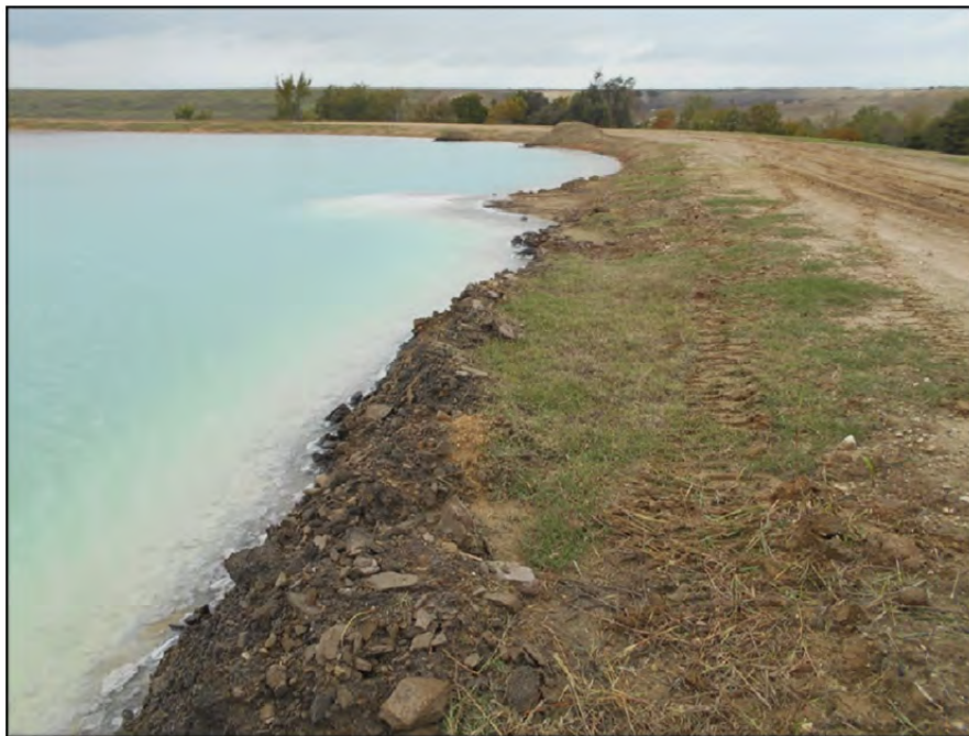
Photograph P-33 – Taken November 11, 2015 by David E. Nielson Secondary E Pond: Looking north from central dike along the inside slope of the eastern dike. The non-linear shoreline is likely a result of dredging activity and not dike instability.
