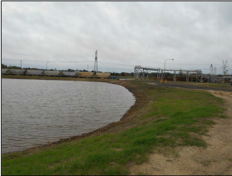
Photograph P-6 – Taken November 11, 2015 by David E. Nielson Pond E: Looking south along west pond interior slope of western edge, which is incised. Note minor vegetation deficiencies, which do not result in significant risk due to incised condition.
