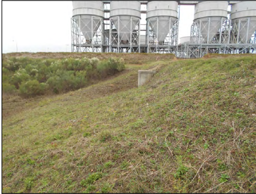
Photograph P-21 – Taken November 11, 2015 by David E. Nielson Pond ST-18: Looking east at outside slope of northern edge of pond. Note the steep dike section in the vicinity of the outlet structure manhole. This dike is steeper than typical. Additional fill should be placed and compacted to lessen the steepness of the slope and increase the dike stability. No evidence of dike instability was noted.
