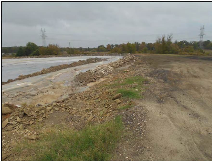
Photograph P-41 – Taken November 11, 2015 by David E. Nielson Secondary E Pond: Looking south at inside slope of western dike and dike crest. Note rigid consistency of excavated stabilized sludge. The Secondary E Pond has significant accumulations of stabilized sludge that promotes stability of the dike system.
