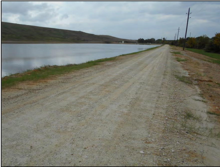
Photograph P-49 – Taken November 11, 2015 by David E. Nielson Pond 002: Looking east along the crest of the southern dike.
