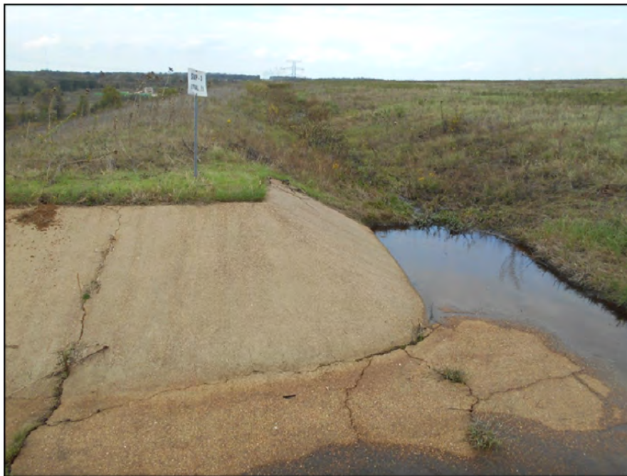
Photograph P-59 – Taken November 11, 2015 by David E. Nielson Landfill Area 5: Looking northwest at stormwater collection ditch at crest of landfill slope where it discharges into concrete lined rundown channel. Note cracks in channel concrete and good vegetation cover. Ponded water is from recent precipitation and not of concern.
