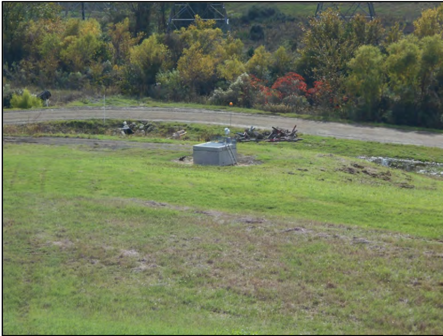
Photograph P-70 – Taken November 11, 2015 by David E. Nielson Landfill Area 9: Looking south at pump station for French drains located at toe of capped landfill slope. Note disturbed vegetation right of pump station (see Photograph P-71).
