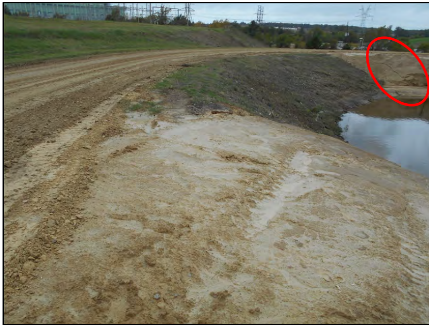
Photograph P-17 – Taken November 11, 2015 by David E. Nielson Pond ST-18: Looking west at inside slope of southern edge of incised portion of pond. Tension crack (circled in red) was in loose CCR material that is to be removed from the pond. No instability of the pond dikes was observed.
