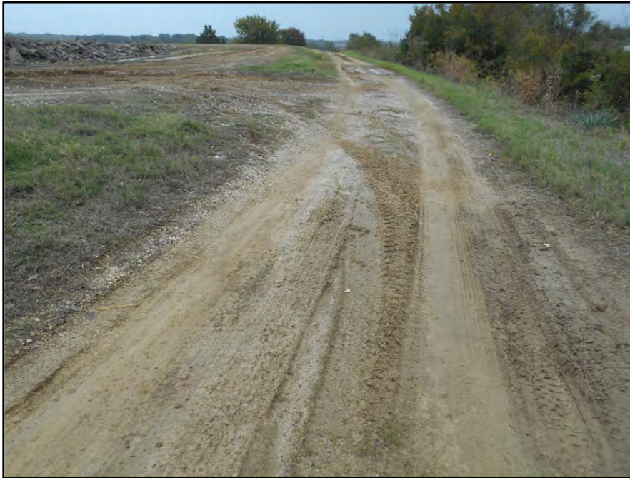
Photograph P-30 – Taken November 11, 2015 by David E. Nielson Secondary E Pond: Looking east along the wide crest of southern dike. Note water ponding in ruts along roadway.
