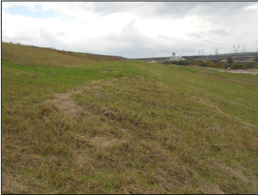
Photograph P-62 – Taken November 11, 2015 by David E. Nielson Landfill Area 5: Looking southeast along the mid-slope bench. Note good slope uniformity and good vegetation cover.
