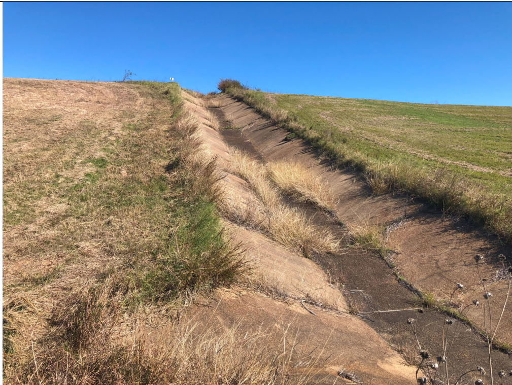
Photograph P-4: View looking east-northeast up the concrete stormwater outfall in Area 5.
