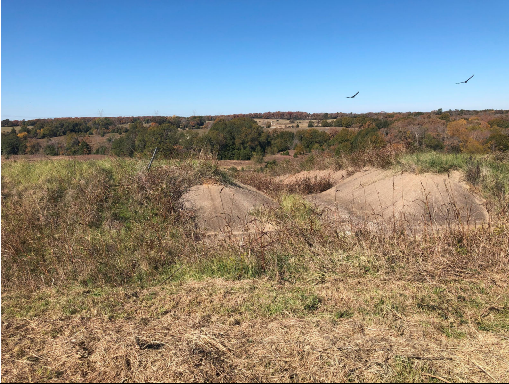
Photograph P-3: View looking west-southwest from Area 5. A stormwater ditch located along the perimeter of the top of the landfill drains to this concrete outfall (also shown in photograph P-4). The ditch appeared to flow well, without significant rutting or standing water.
