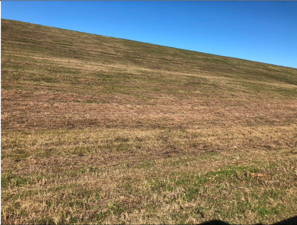
Photograph P-6: View looking north up the side slope of Area 9. The terraced slope is well vegetated with no visible sloughing or erosional issues.
