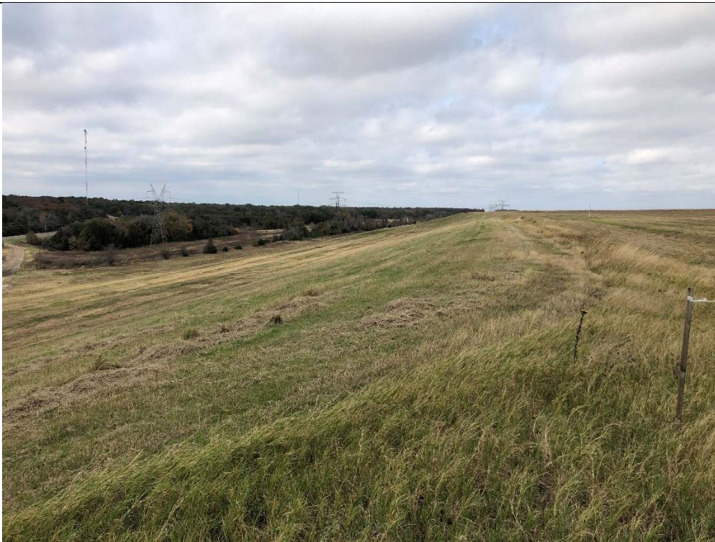
Photograph P-6: View looking northwest along Area 9 side slope. The slope is well vegetated with no visible sloughing or erosional issues.
