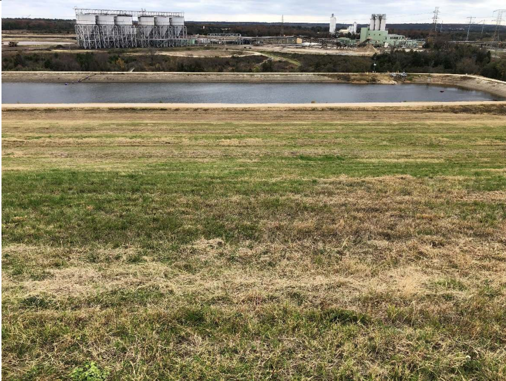
Photograph P-5: View looking south-southeast across down the side slope of Area 9 and across Pond 002. The slope is well vegetated with no visible sloughing or erosional issues. Pond 002 is a stormwater pond where contact stormwater is managed.
