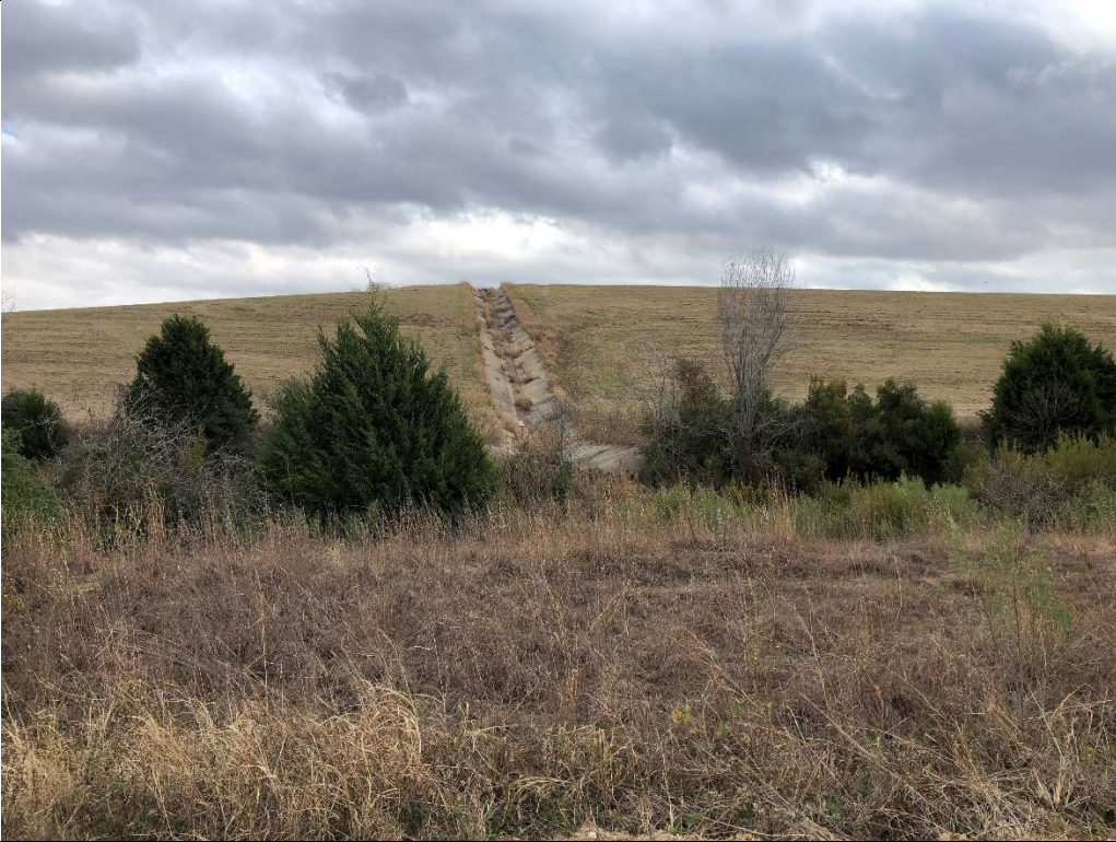
Photograph P-11: View looking southeast at the concrete drainage structure located in Area 1. The slope is well vegetated with no visible sloughing or erosional issues.
