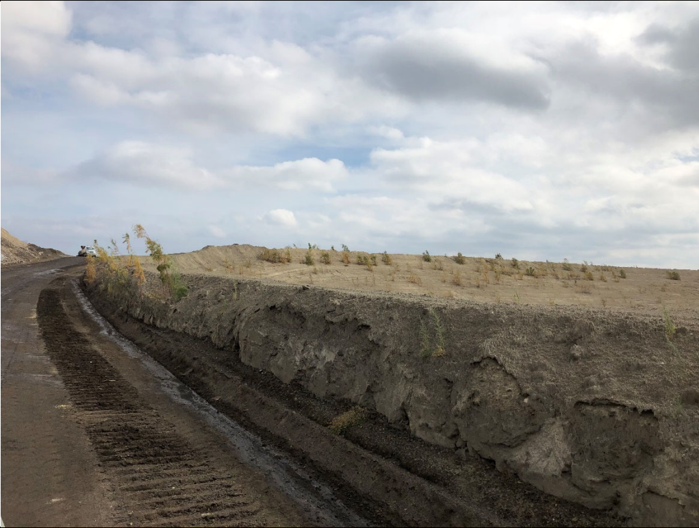
Photograph P-7: View looking east at uncapped CCR waste material and a CCR material berm/sidewall in Area 7. One of the landfill haul roads (improved with bottom ash) with no significant rutting is visible to the left. As evidenced by the sheer sidewall visible here, the CCR waste is a rigid material.
