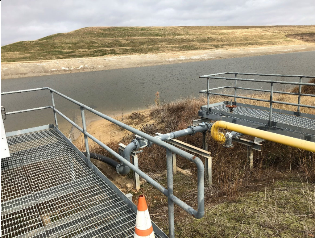
Photograph P-5: View looking north from equipment skid across Pond 002 at sidewall of the Unit 004 Landfill. The sidewalls of Areas 9 and 10 are visible in this photograph.
