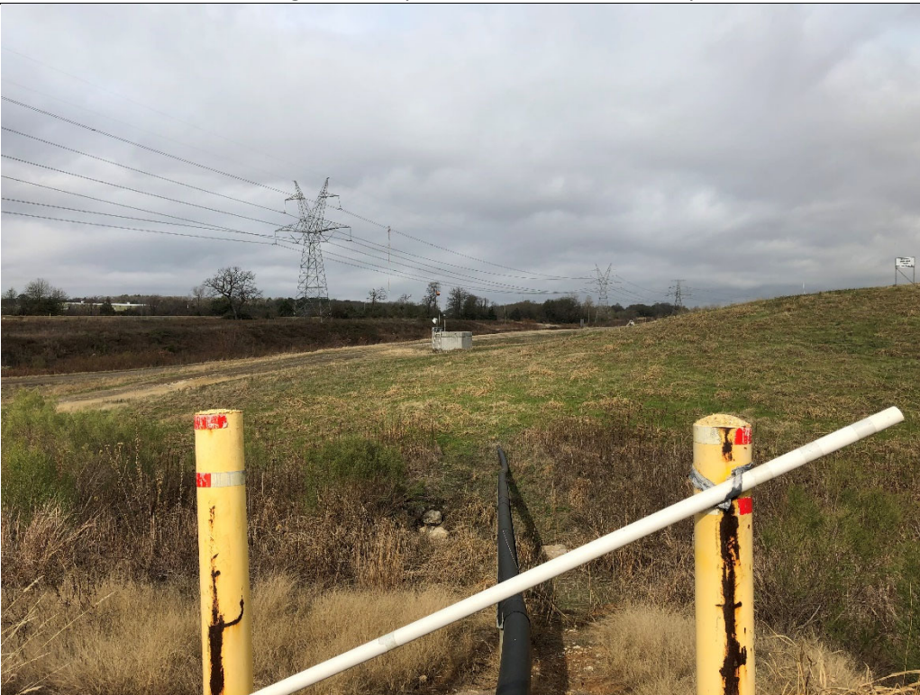
Photograph P-4: View looking north-northwest of sump on southwest corner of Unit 004 Landfill. A French drain system empties into the concrete sump, which is then pumped through the black pipe (bottom center) into Pond 002.
