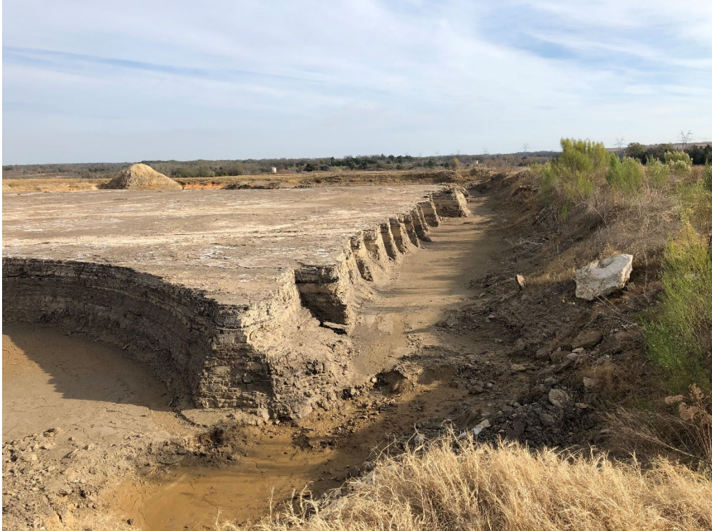
Photograph P-12: View looking east-northeast of the northern half of the Unit 003 Secondary E Pond. The central, separating berm is visible on the right and the rigid stabilized waste material is visible on the left. The waste has been partially excavated from the perimeter of this portion of the pond. The stockpile (left background) is CCR waste material stockpiled inside of the pond.
