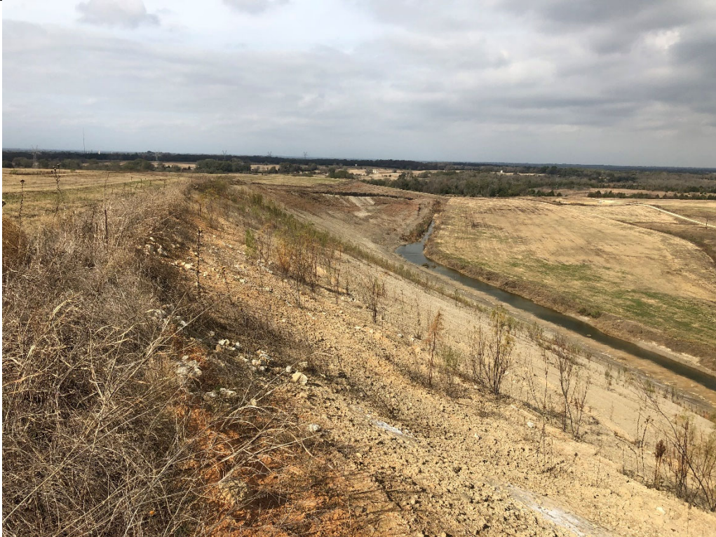
Photograph P-6: View looking northwest of sidewall of Area 4. The top of this area (far left of photograph) is capped. The sidewall of Area 4 (center of photograph) is not capped. The exposed waste is rigid CCR waste. The contact water interceptor ditch is visible on the right side of the photograph. Area 17 is visible to the right of the interceptor ditch.
