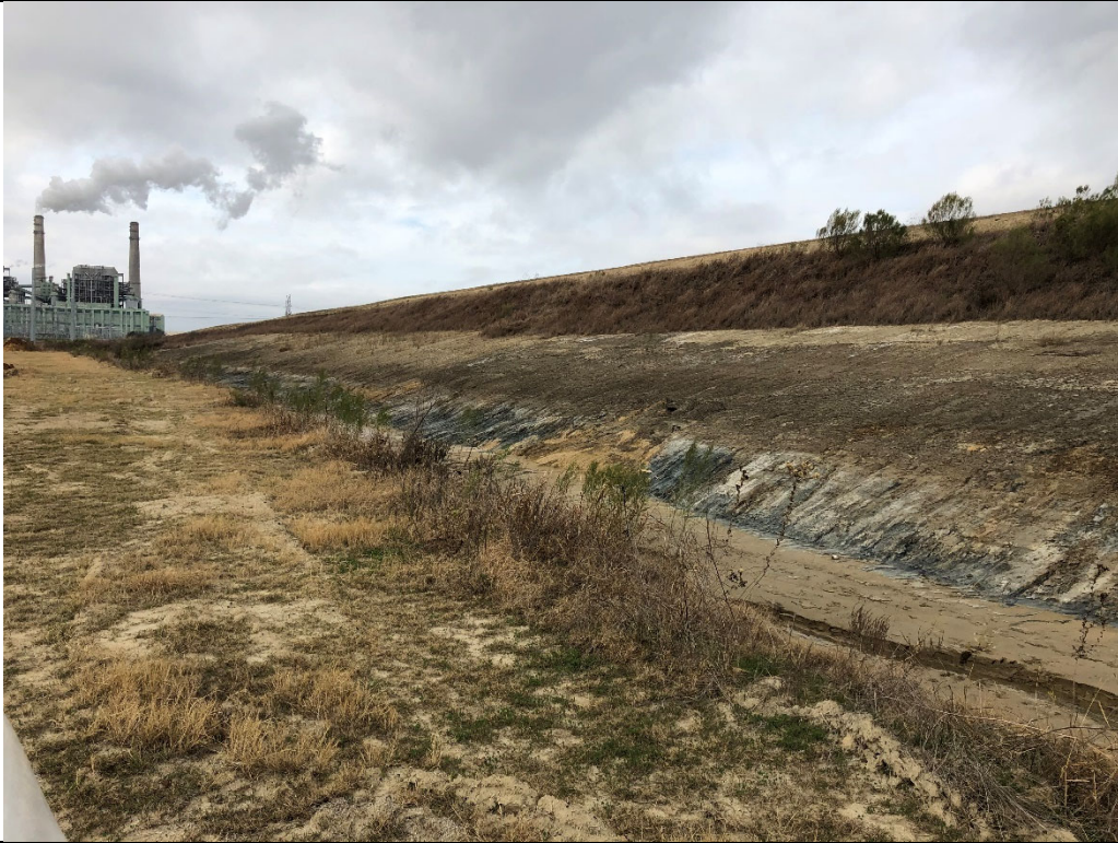
Photograph P-11: View looking west of CCR contact water interceptor ditch. The sidewall of Area 10 is visible on the right side of this photograph. The sidewall is either well vegetated or stabilized to prevent erosion.
