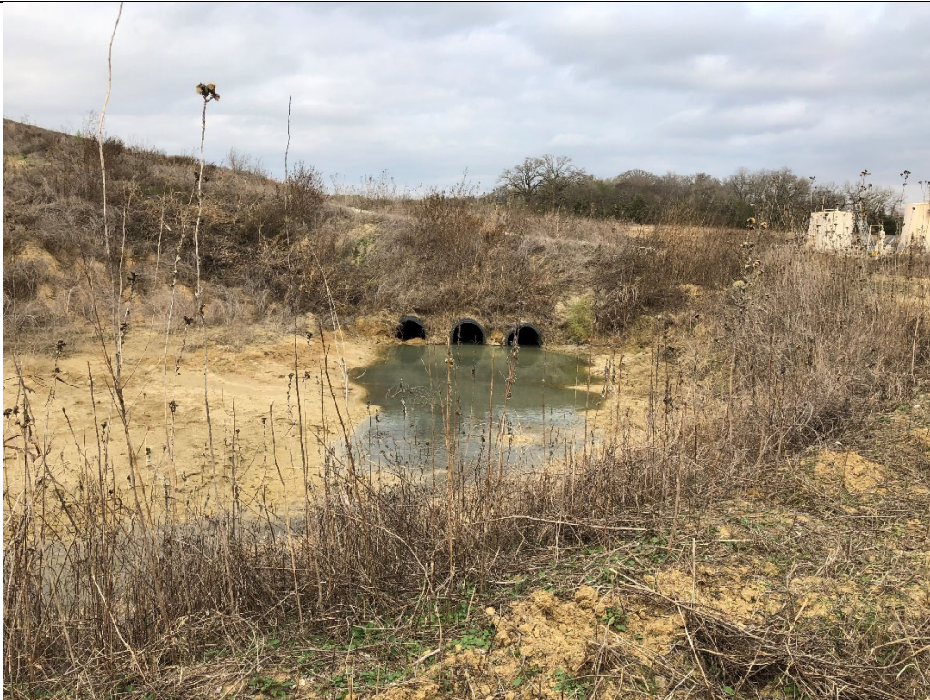
Photograph P-10: View looking east-northeast of CCR contact water interceptor ditch. The interceptor ditch is bridged in this location by a second drainage feature that conveys stormwater from the capped portion of Area 8 to the non-contact water drainage ditch.
