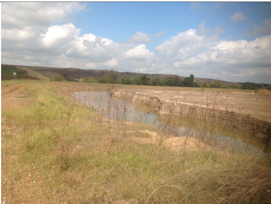
Photograph P-13 Taken November 6, 2018 by Jason Leik, P.E. Unit 003 Secondary E Pond – Looking north along top of and interior of west berm
